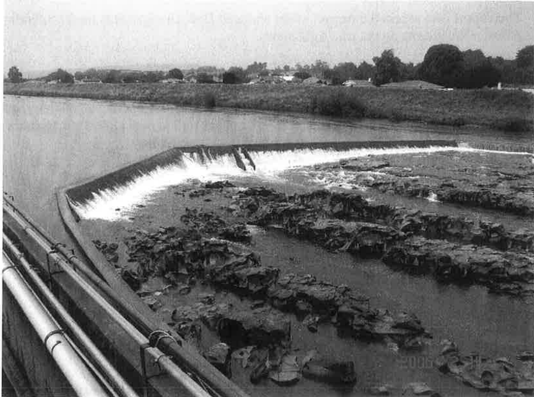
Figure 2: Photo of weir shows fish pass in centre from Alliance (right side) bank. Estimated total river flow above weir is 23 m 3 /s at 1100 hrs 14 Feb 2006
