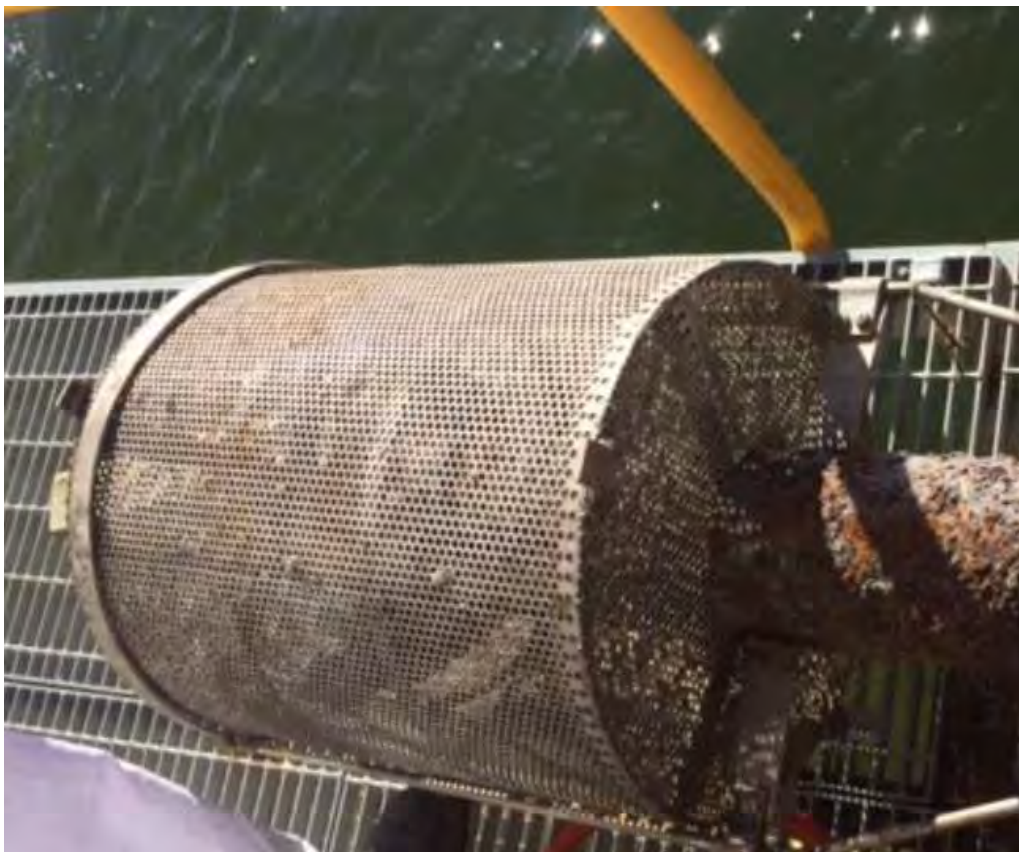
Figure 4: Screen on one of the intake pumps within the hydro race.
