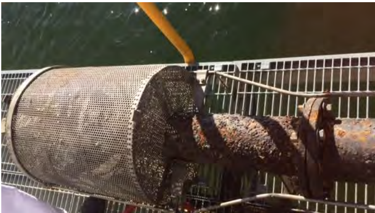
Figure 54: View of the intake pumps located within the hydro-race.
