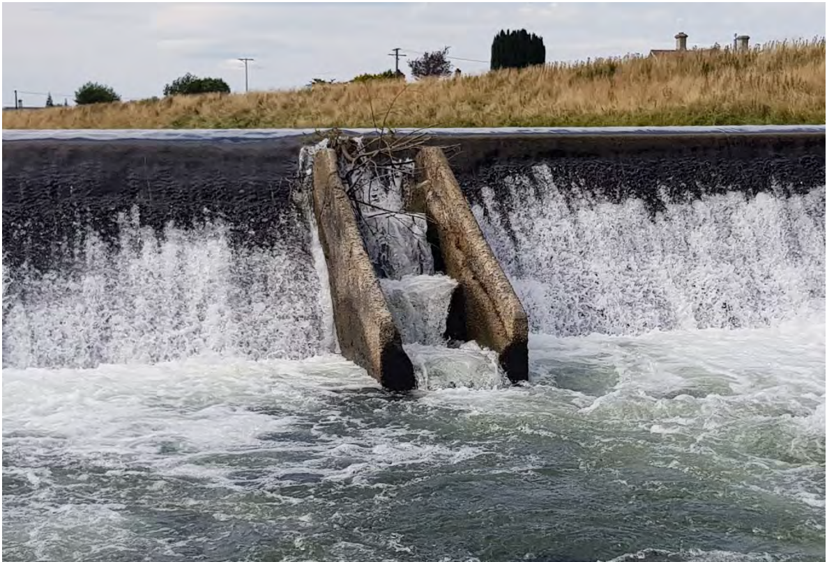
Figure 4. Close up of the fish ladder showing debris caught at the top of the weir.
