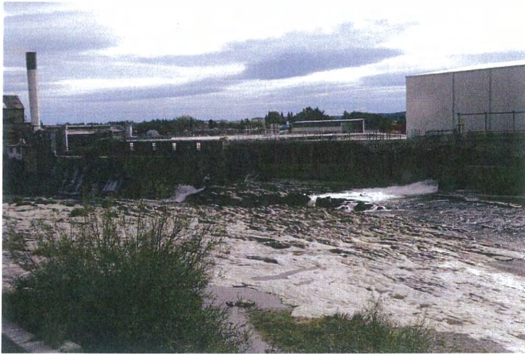
Figure 6. Alliance Matura showing flows from the headrace through sluice gates and overflows
