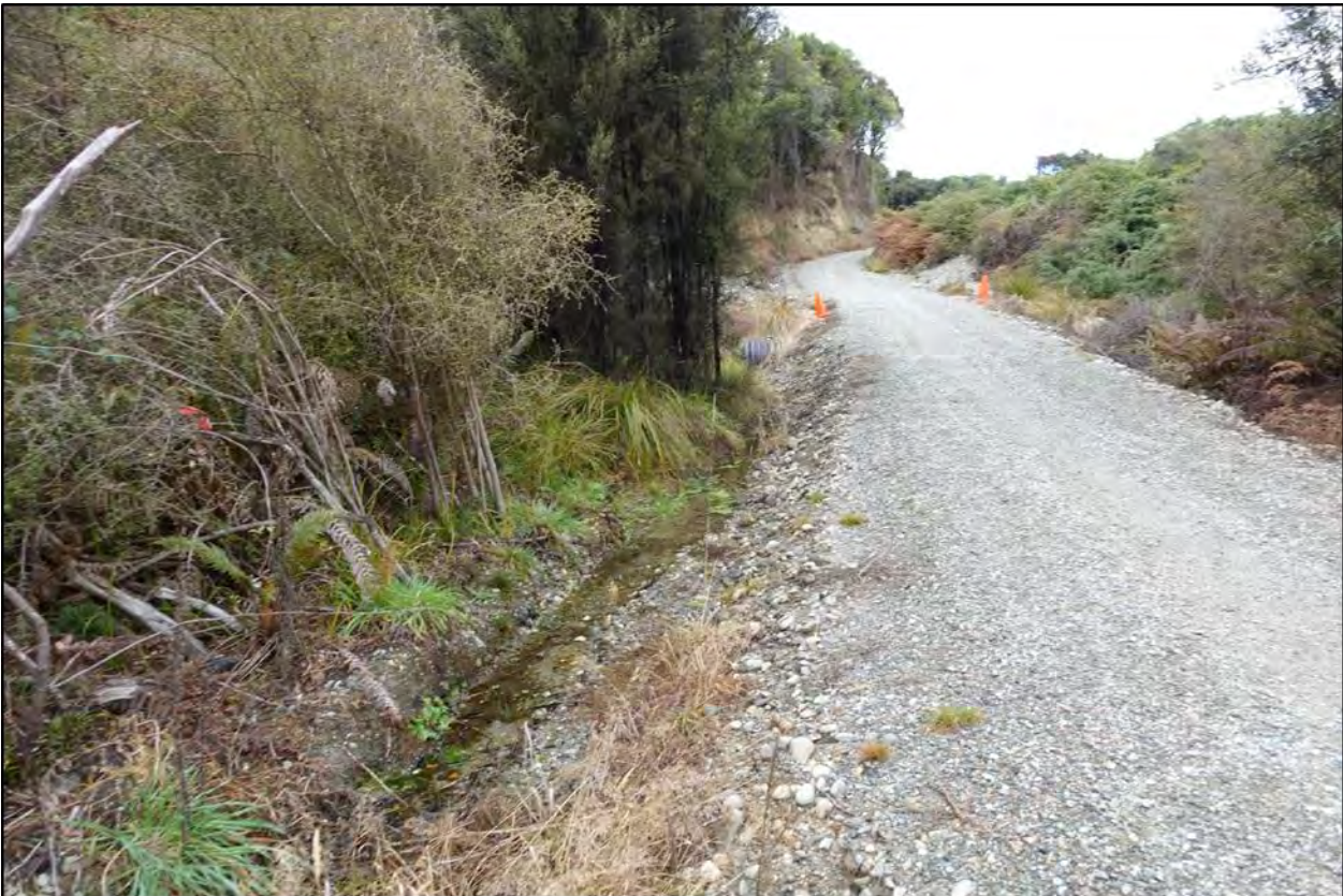
Small water table formed to direct sub-surface and small surface flows into the southern culvert (visible by orange road cone).
