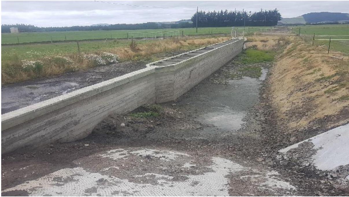
Figure 18: Sludge bed/weeping wall at SD1 constructed in 2017
