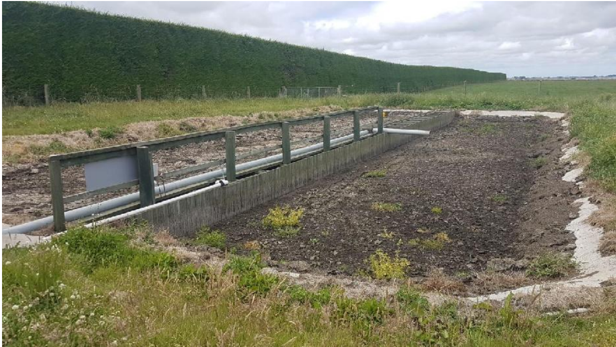
Figure 20: Sludge bed/weeping wall structure on SD2
