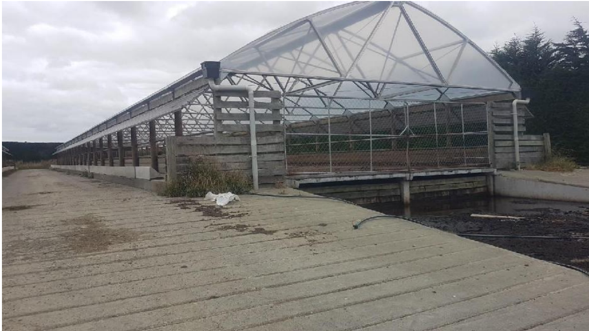
Figure 12: Wintering shed with underground concrete bunkers and weeping wall at front on SD2 and showing uncovered central feed lane
