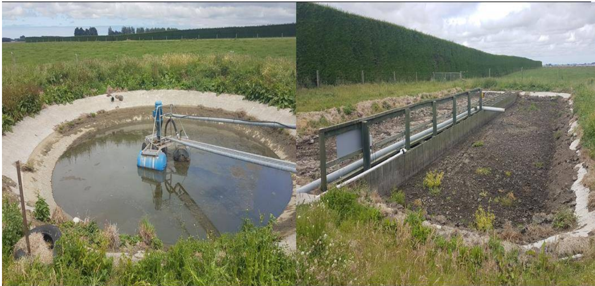
Figure 11: Concrete saucer and sludge bed/weeping wall at SD2
