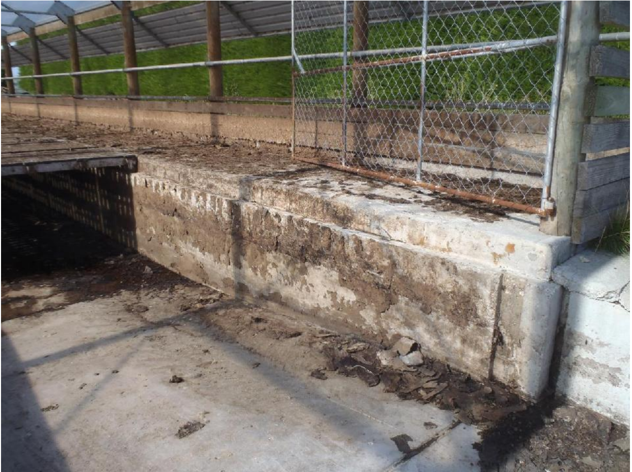
Looking south east at the south wall precast panel with a top slab that holds the removable panels in place.
