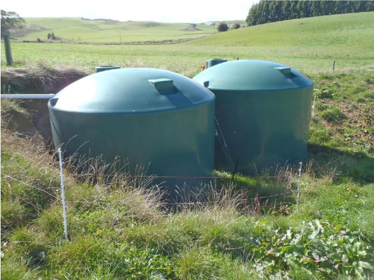
The storage tanks that capture the liquid via a subsoil system under the bunkers.
