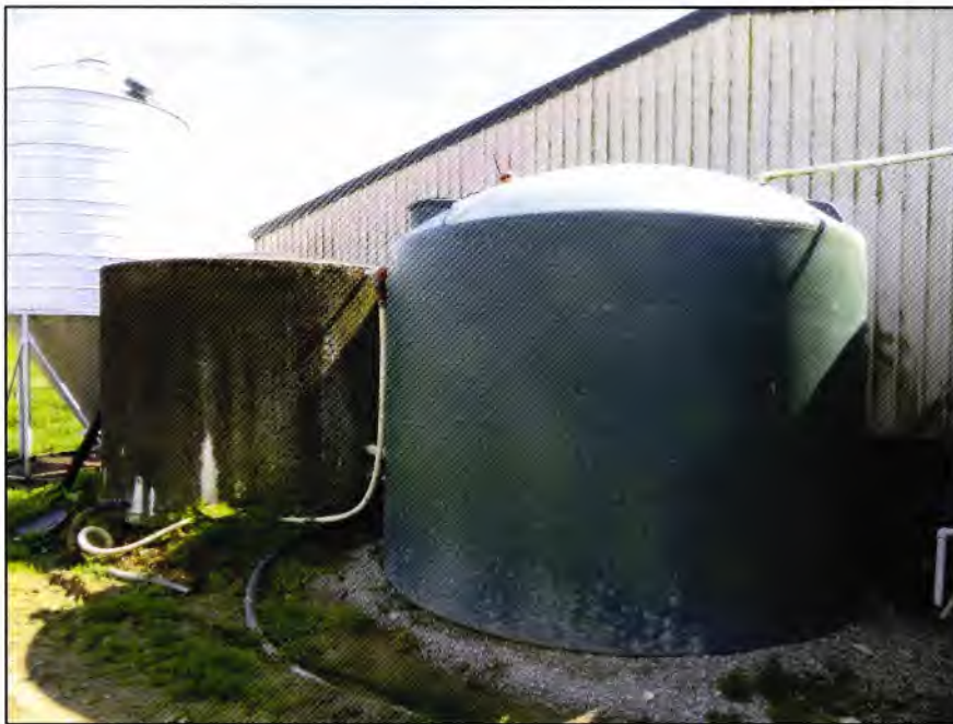
Figure 6.7 two water storage tanks at dairy shed.
