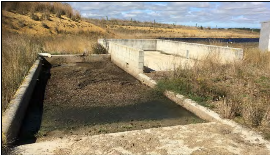
Figure 3: Large stone trap adjacent the effluent pond
