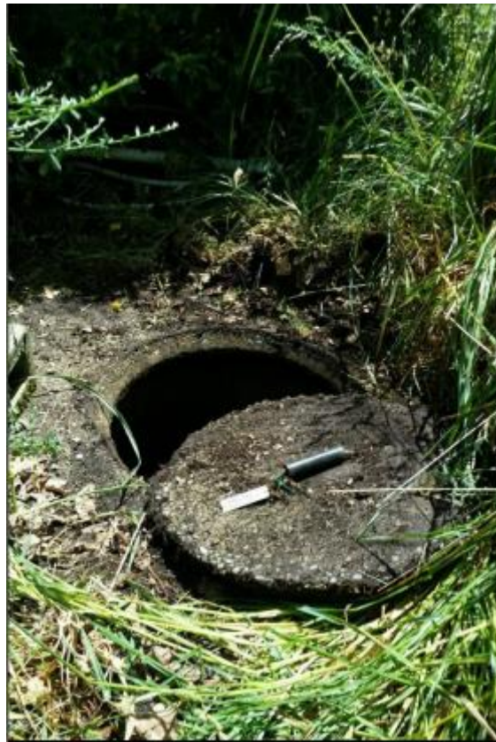
Figure 15: Bore E45/0622 in early 2019, showing the lack of wellhead protection and potential for surface water runoff entry
