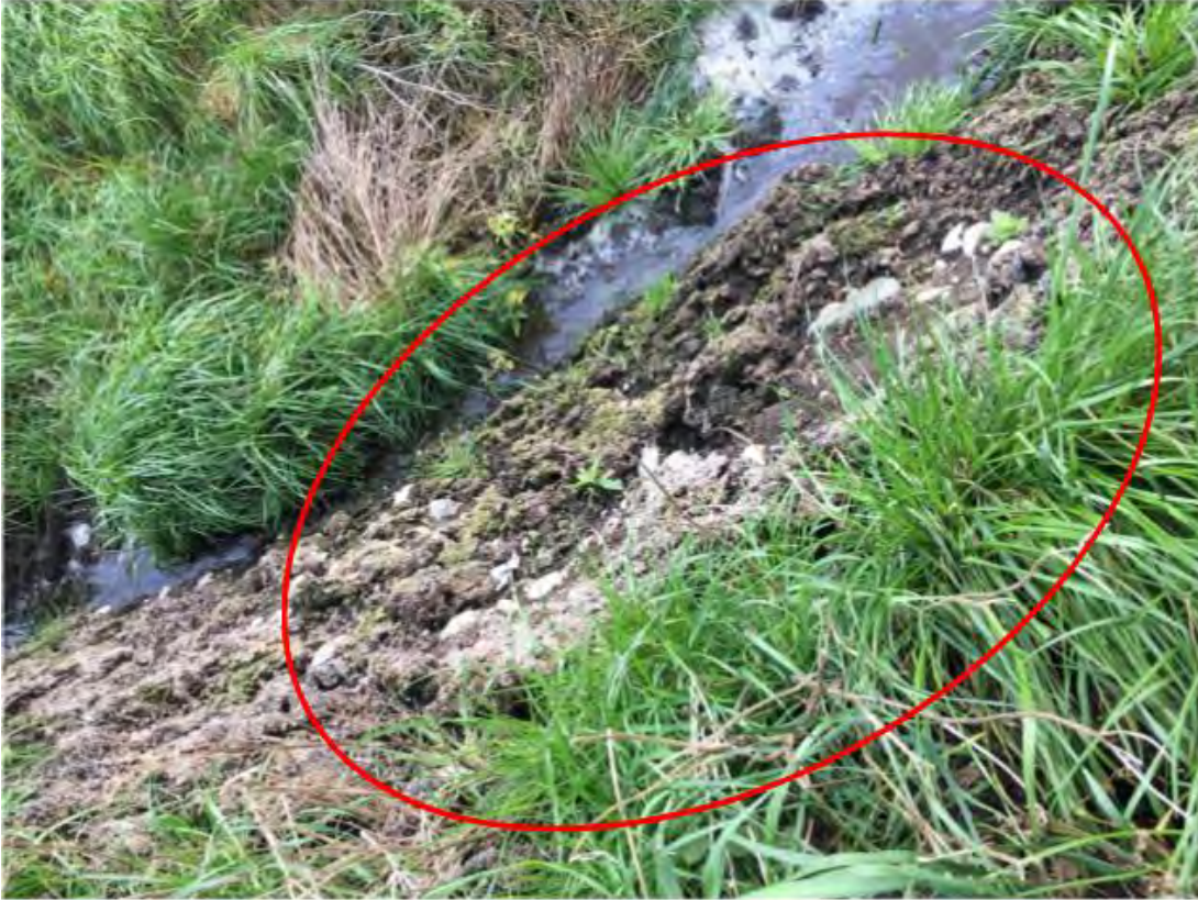
Figure 5.13.4: Rocks visible protruding from pond liner indicating erosion of the liner
