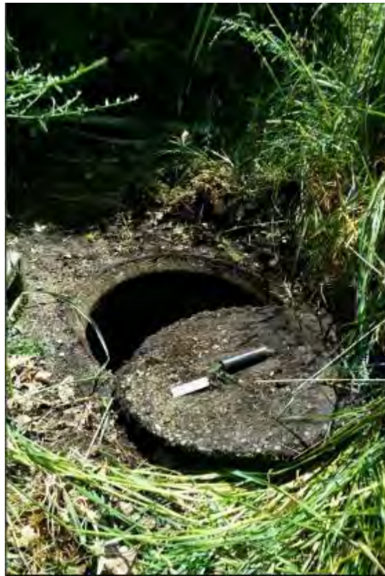
Figure 15: Bore E45/0622 in early 2019, showing the lack of wellhead protection and potential for surface water runoff entry
