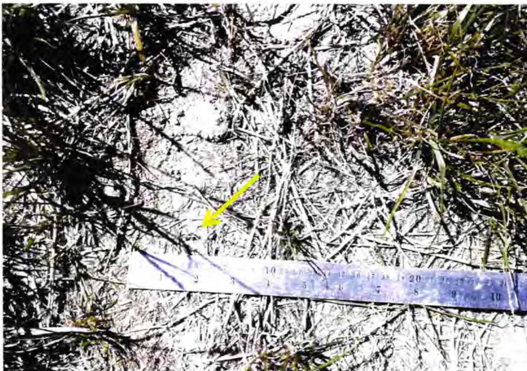
Figure 6. Cracking at Site 3. These cracks do not show up well in the photo because of their smaller size and the high contrast shadows but were easily visible at the time.
