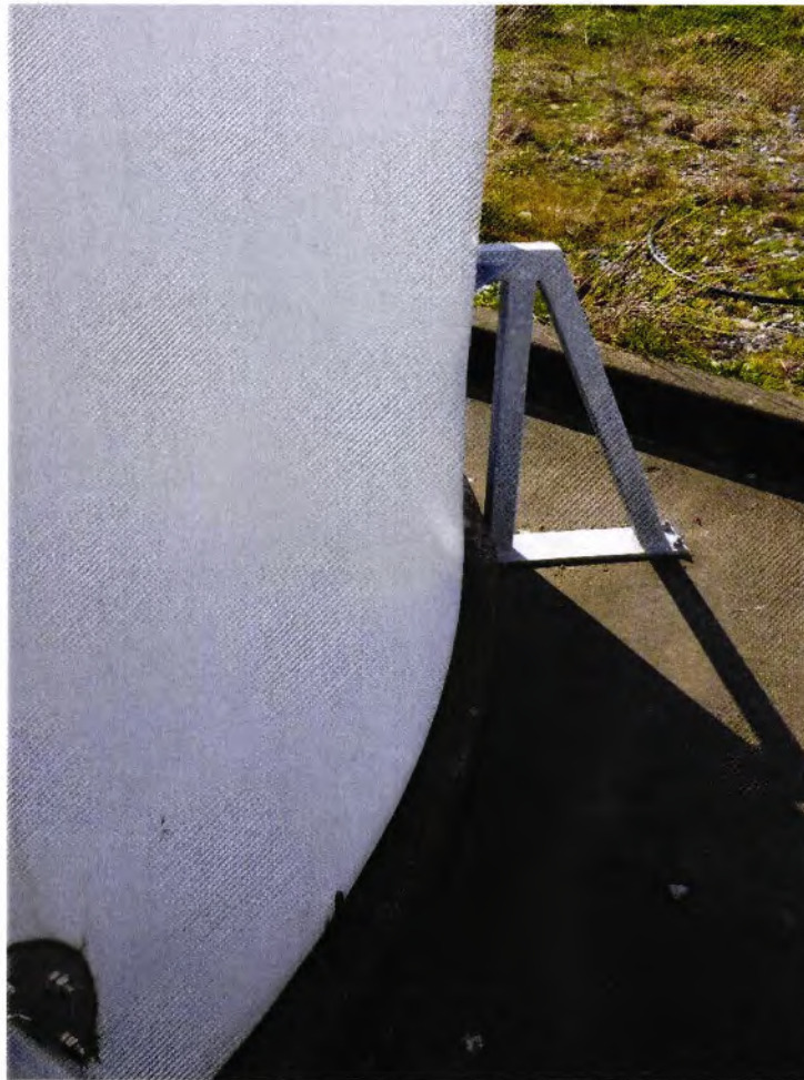
Minor Bulging of Lower Side Wall
