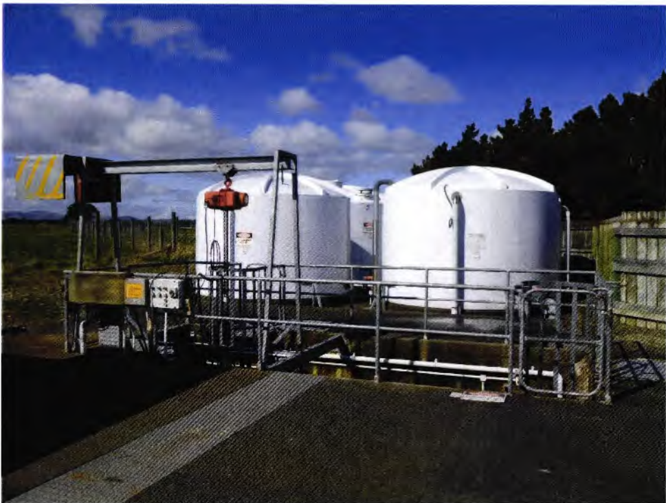
Overall View of Primary Treatment Plant
