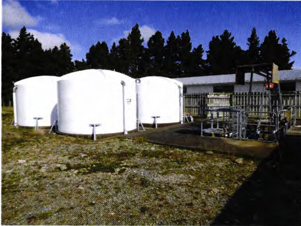
Overall View of Primary Treatment Plant
