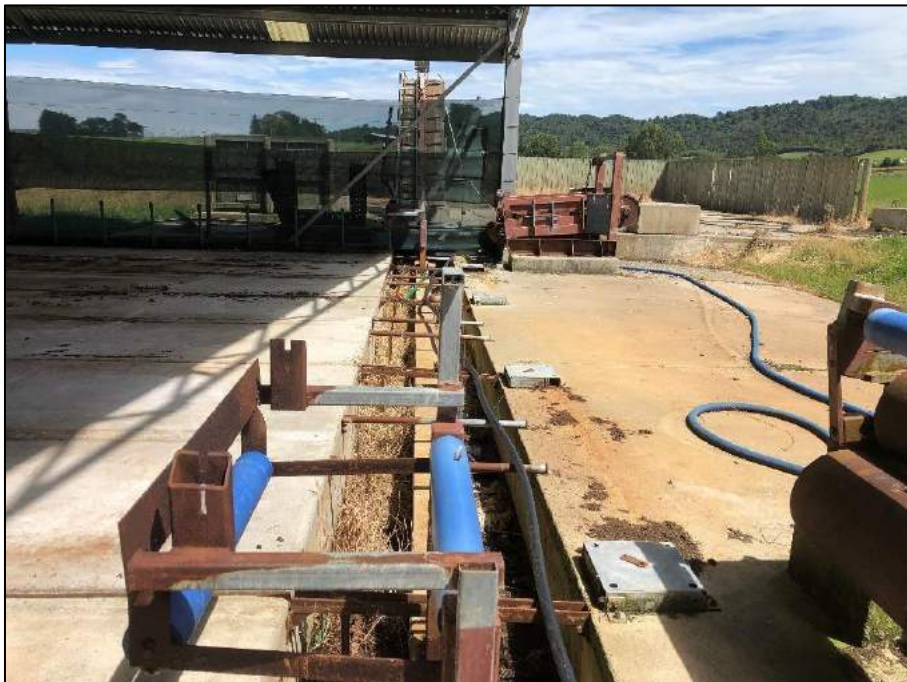
Figure 2.3: Conveyor chain and weeping wall.
