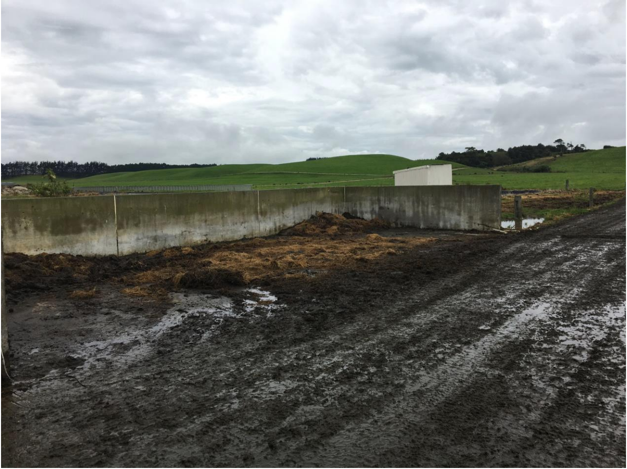
Picture 5: Solids bunker, and liquid effluent flow back into the transfer sump.
