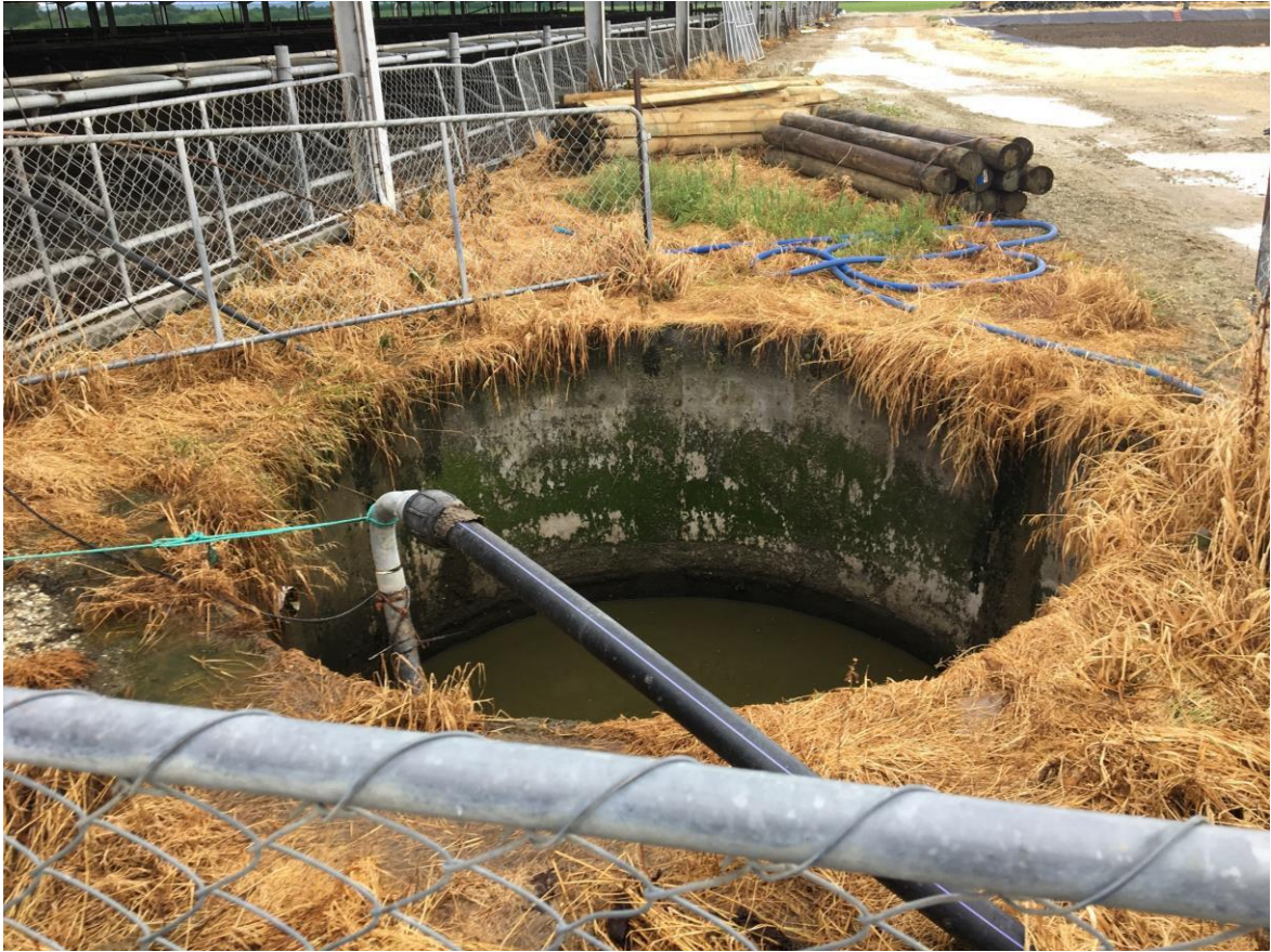
Picture 3: Transfer sump located at the southern entry to the wintering barn.
