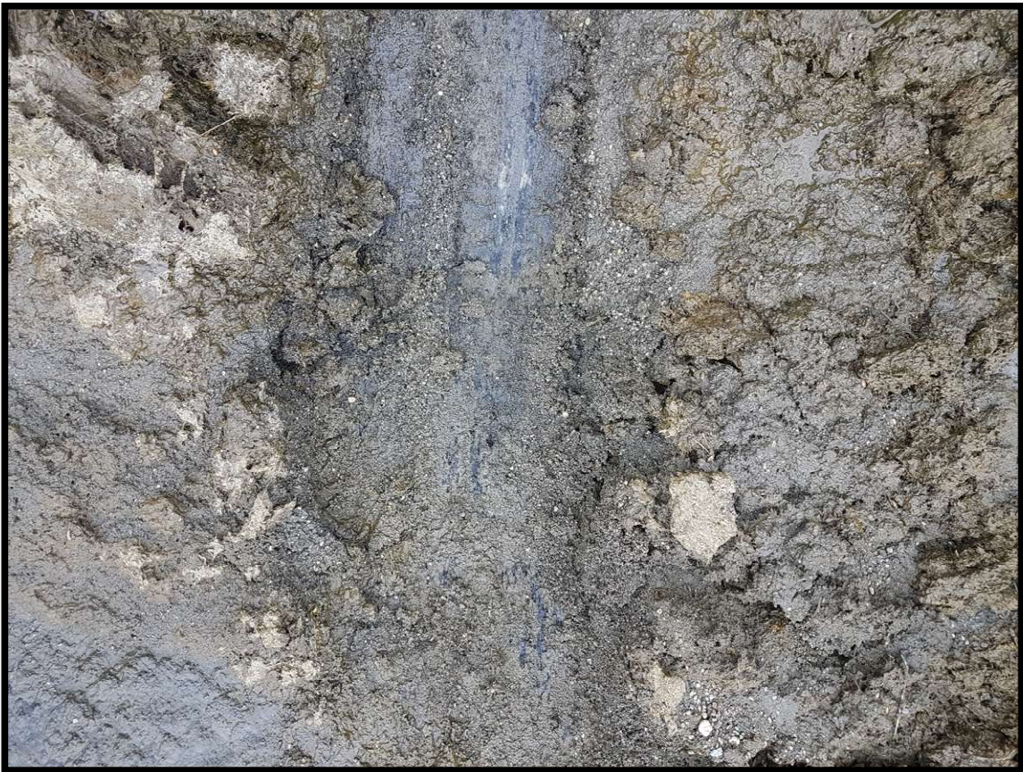
Figure 5 : Area of effluent scraped to reveal the concrete liner
