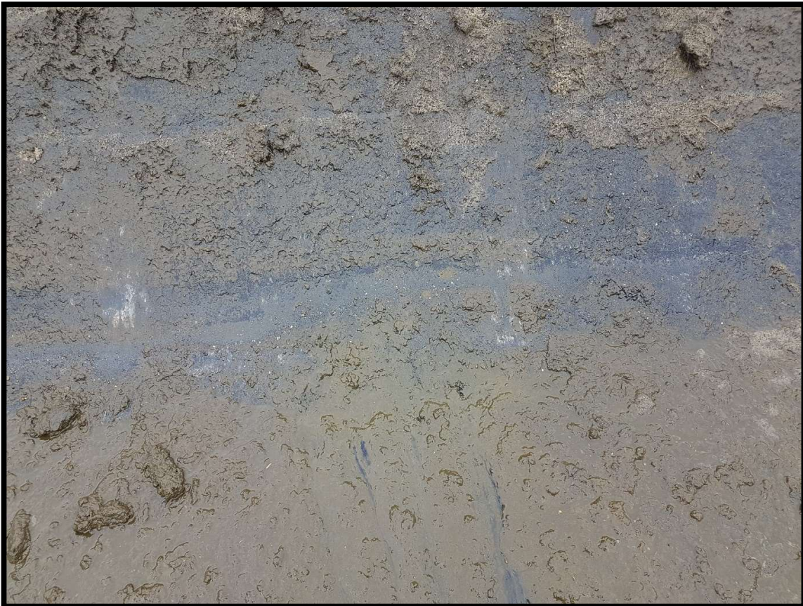
Figure 7 : Scrape mark on embankment
