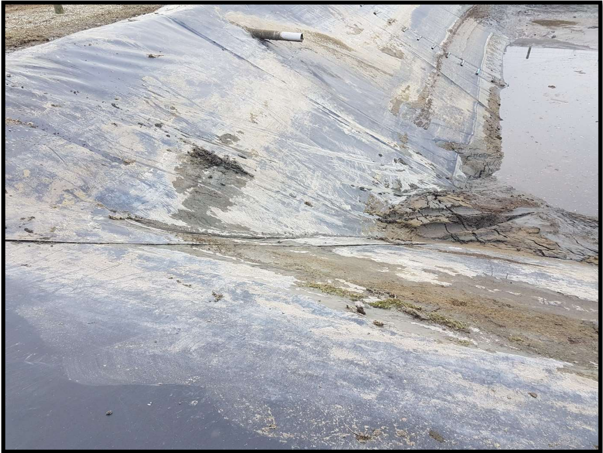
Figure 9 : Inlet Pipe with Additional Liner Protection
