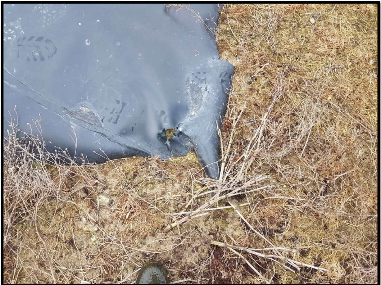
Figure 10 : Liner Rip/Tear Located on Anchor Trench
