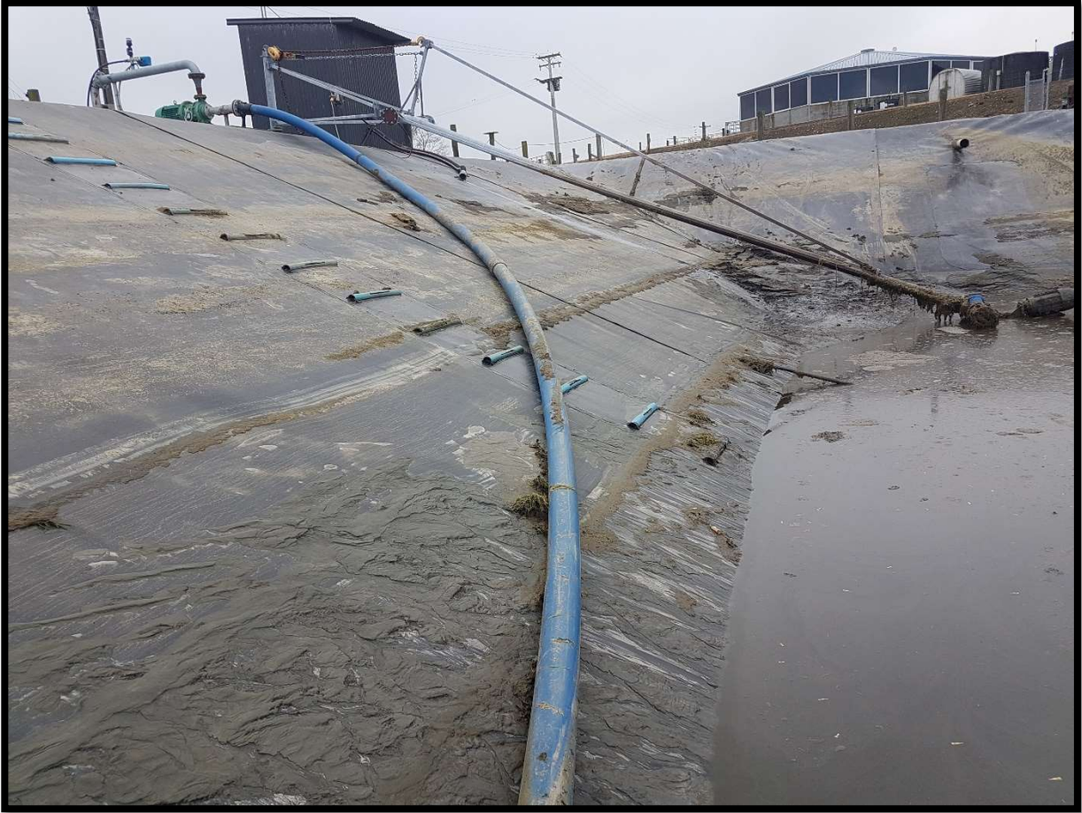
Figure 5 : West Embankment, Pump and Stirrer
