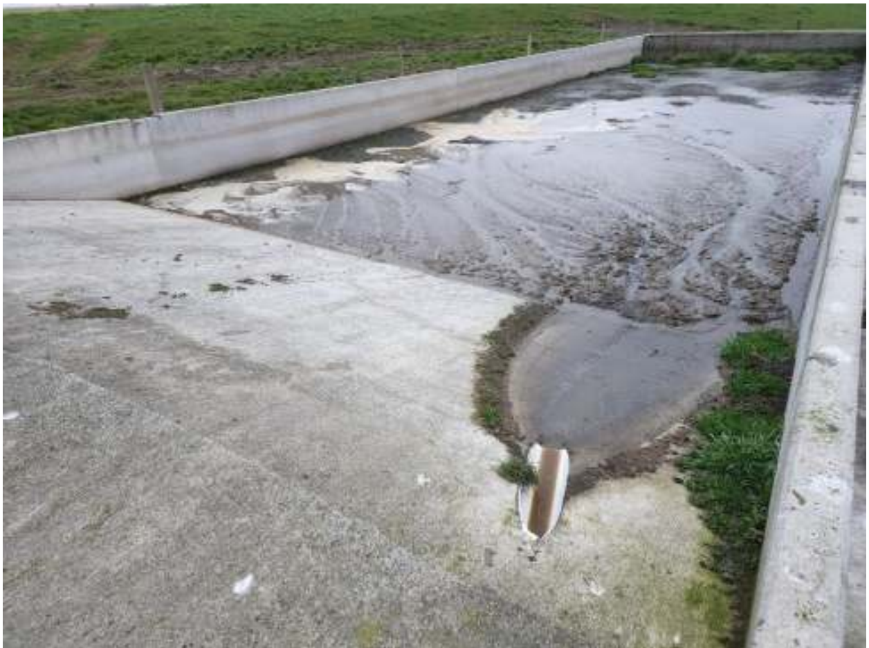
Figure 9 South sludge bed.
