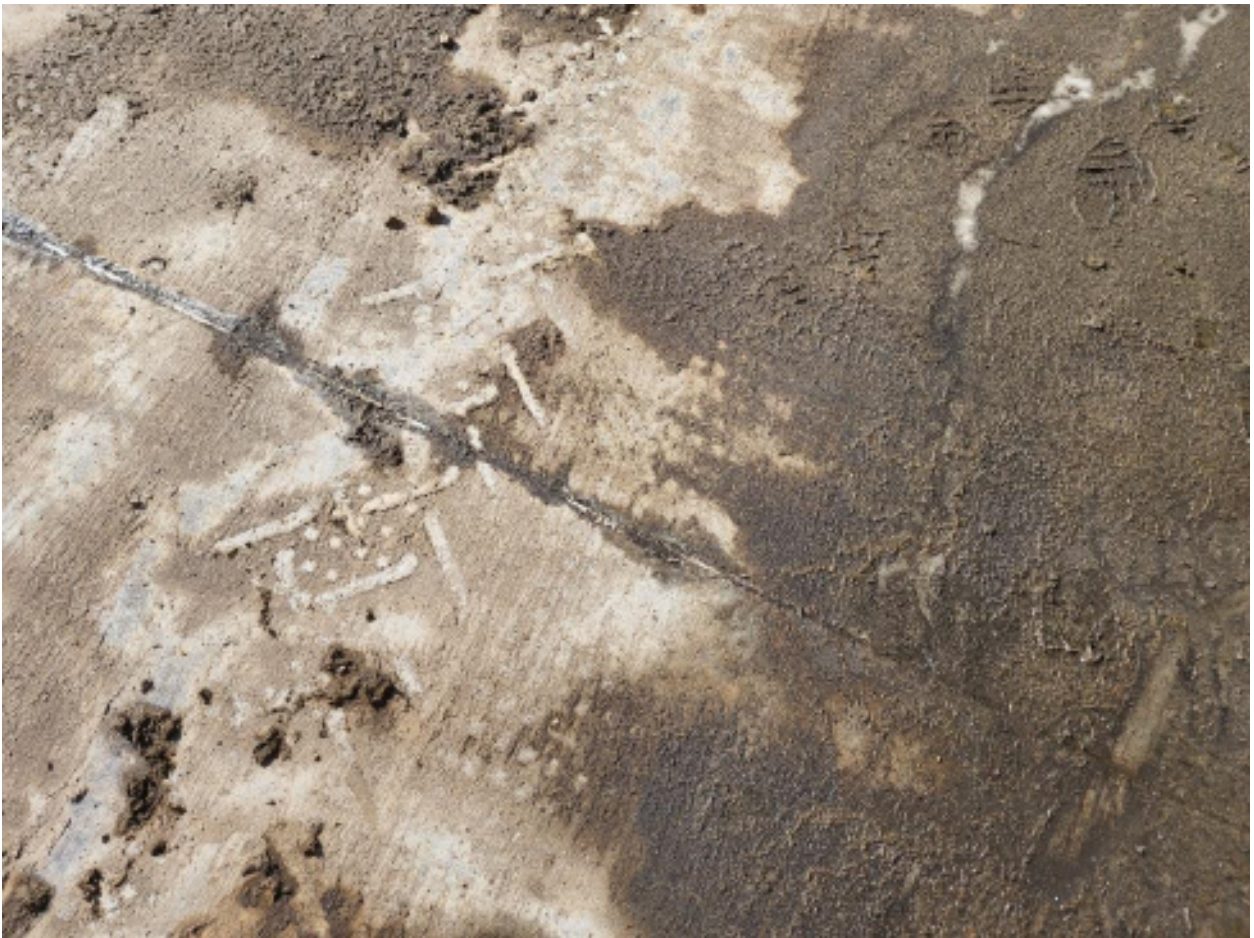
Figure 39 Floor joint of south sludge bed.
