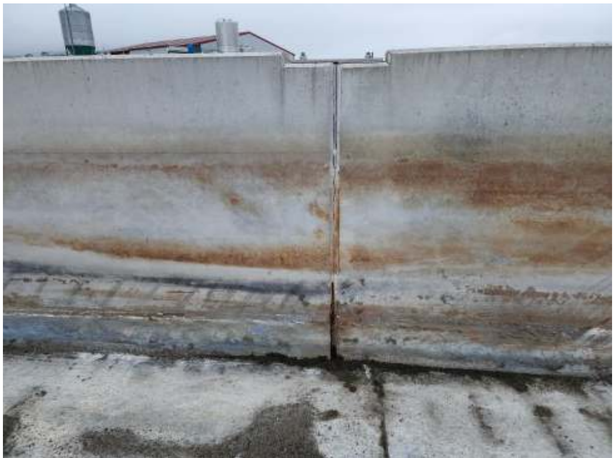
Figure 13 Panel joints of north sludge bed with damage sealant.
