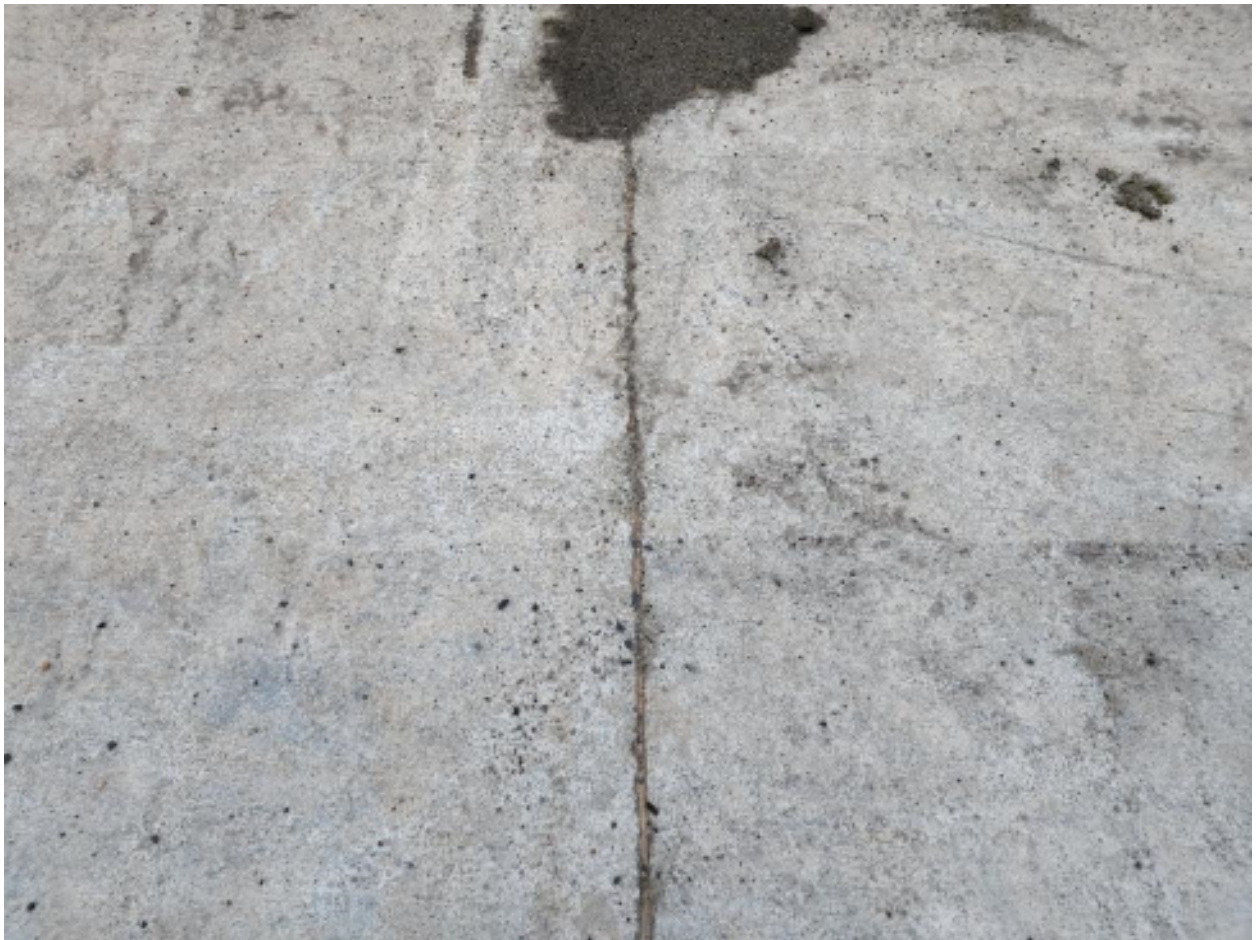
Figure 14 Floor joints of north sludge bed.
