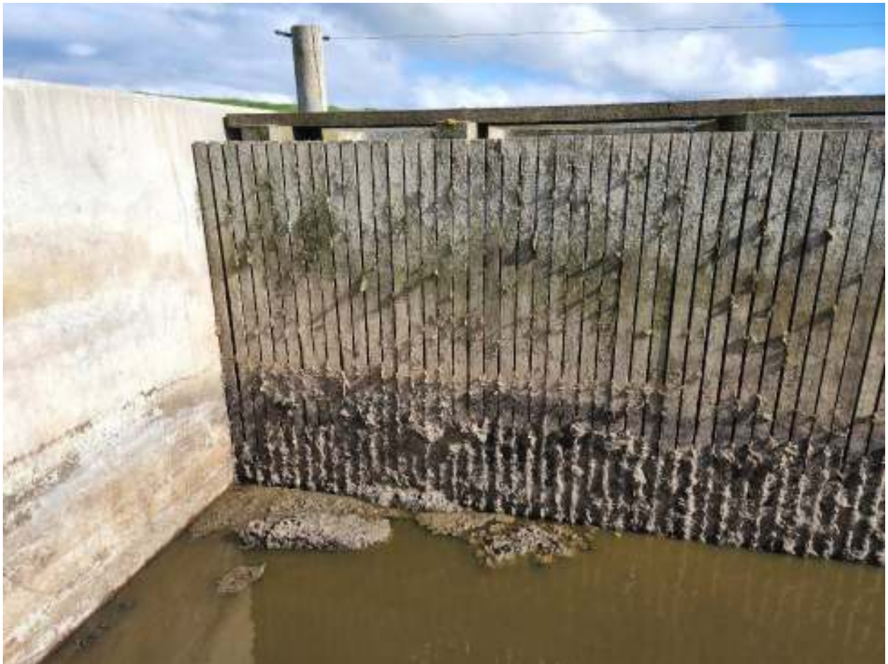
Figure 47 Weeping wall of south sludge bed.
