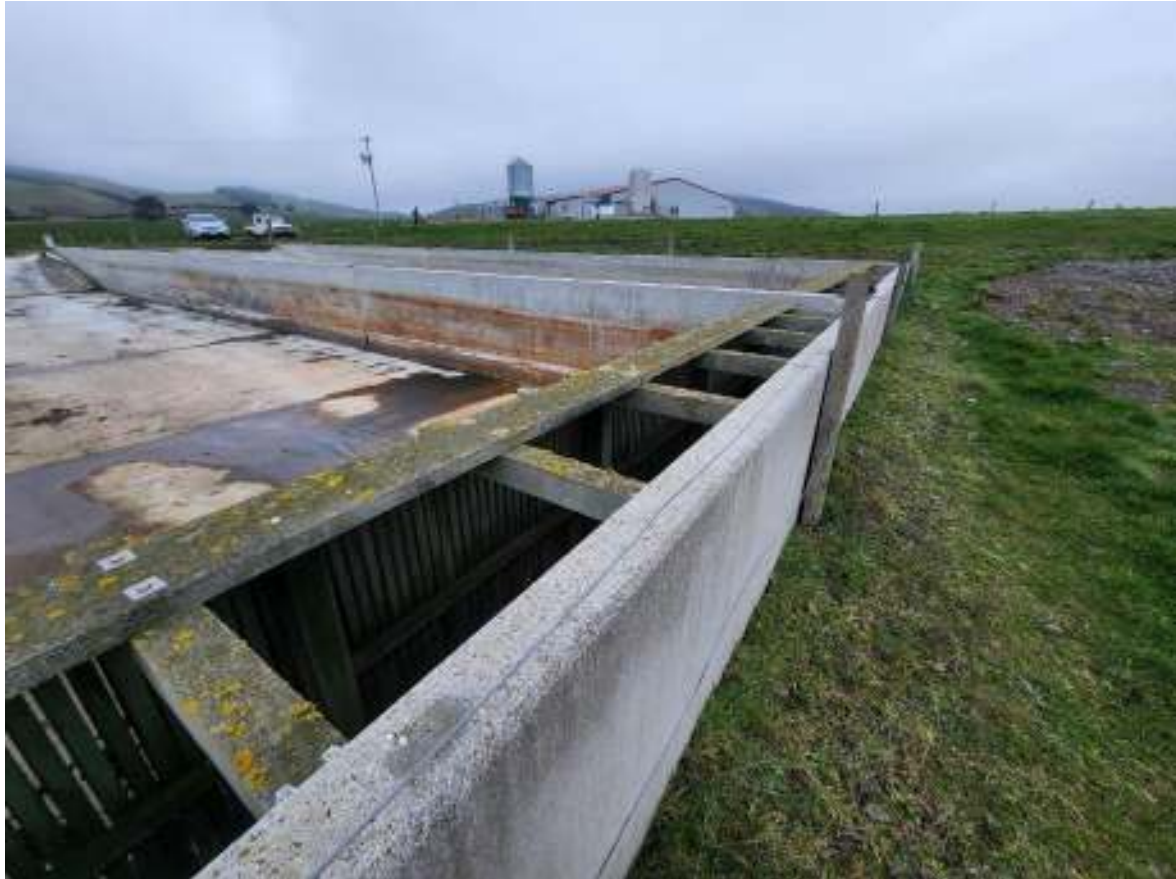
Figure 2 Weeping wall structure and exterior of facility.
