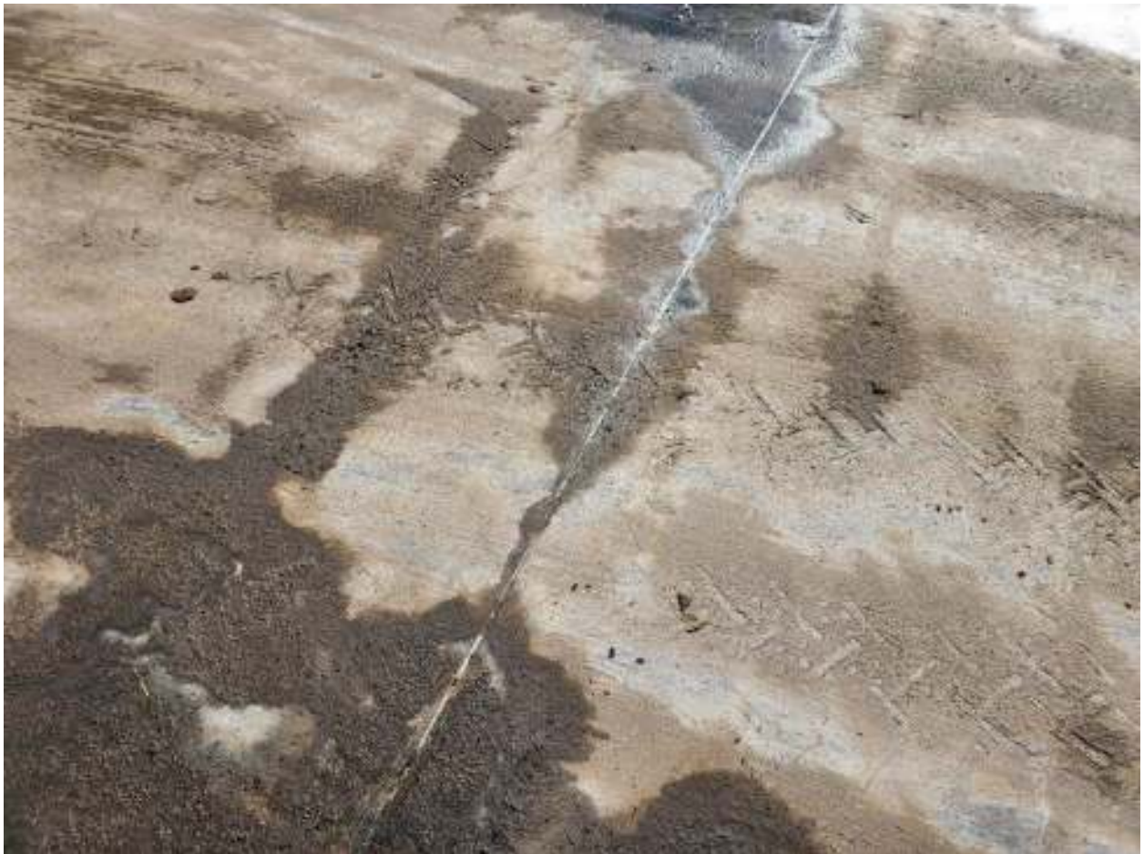
Figure 43 Edge joint of south sludge bed.
