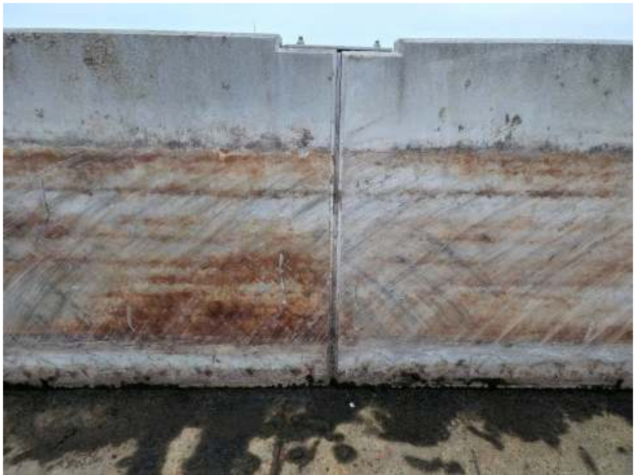
Figure 12 Panel joints of north sludge bed.
