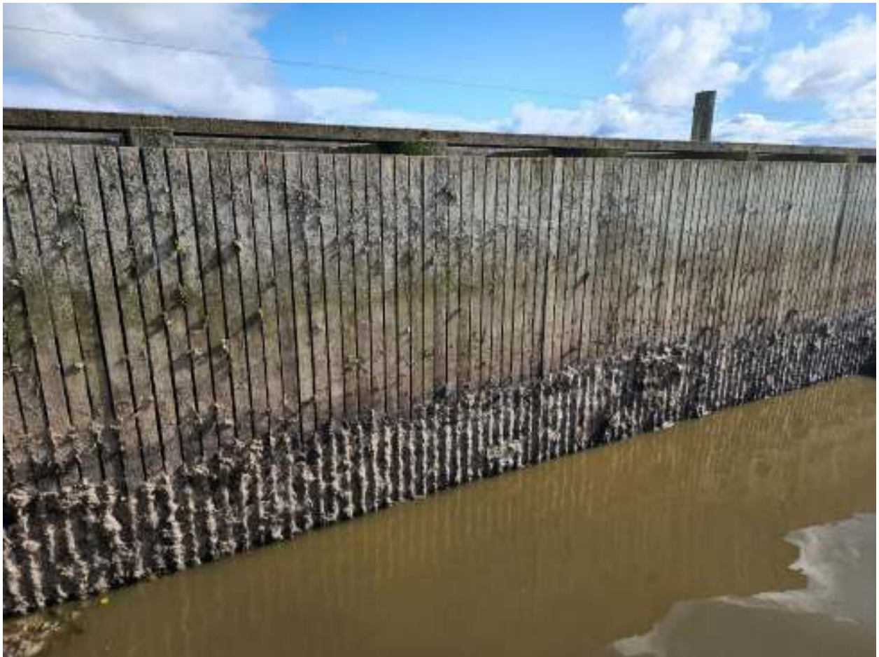
Figure 48 Weeping wall of south sludge bed.
