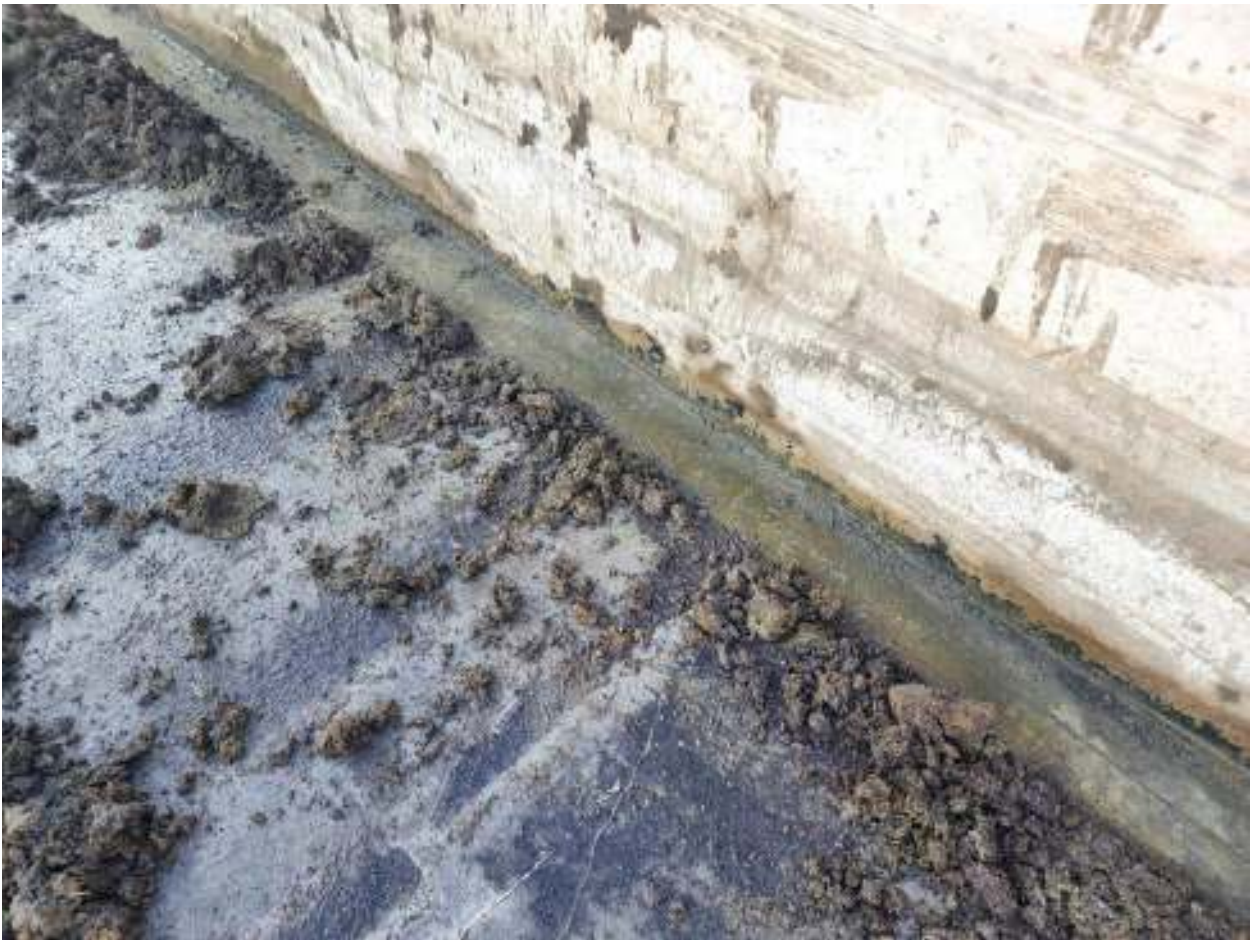
Figure 45 Edge joint of south sludge bed.
