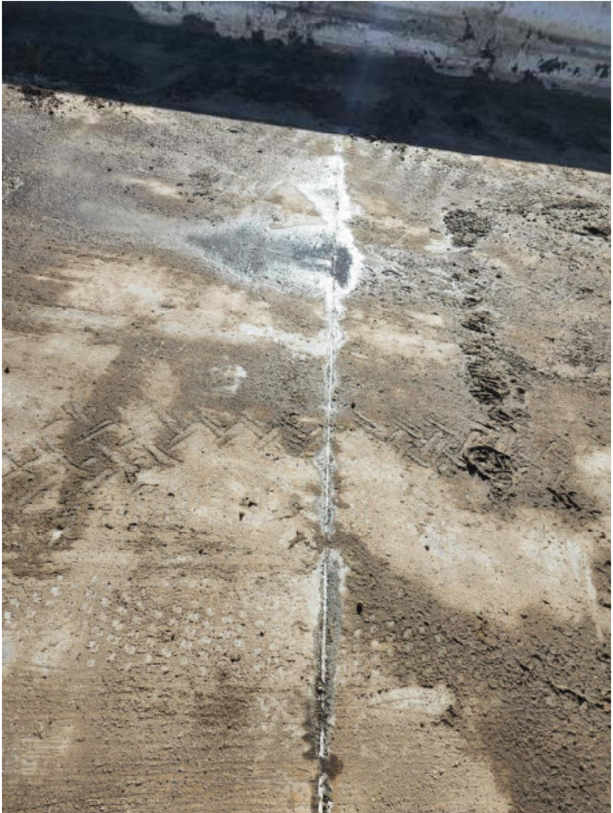
Figure 40 Floor joint of south sludge bed.
