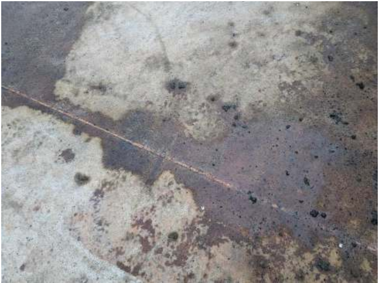
Figure 16 Floor joints of north sludge bed.
