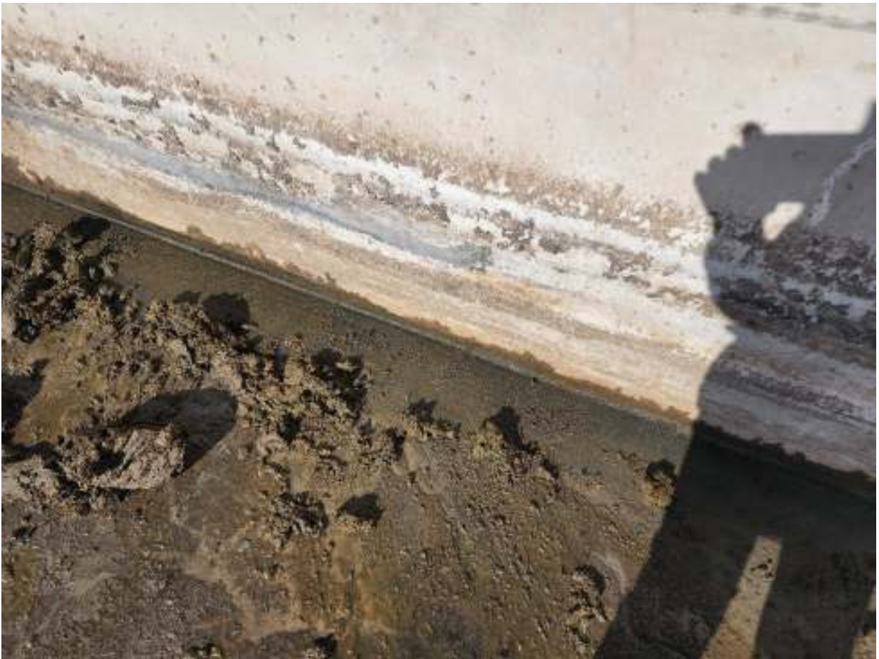
Figure 38 Edge joint of south sludge bed.
