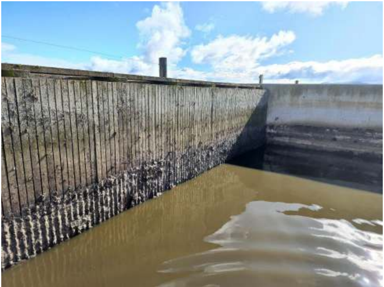
Figure 49 Weeping wall of south sludge bed.
