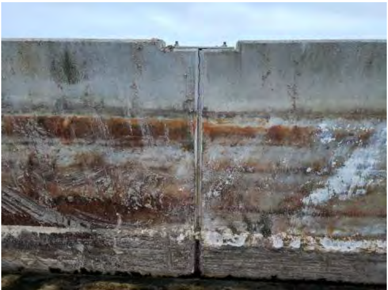
Figure 15 Panel joints of north sludge bed with damaged sealant.
