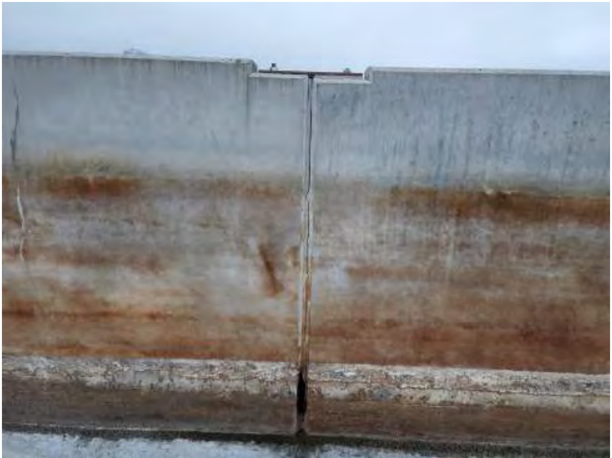
Figure 20 Panel joints of north sludge bed with damaged sealant.
