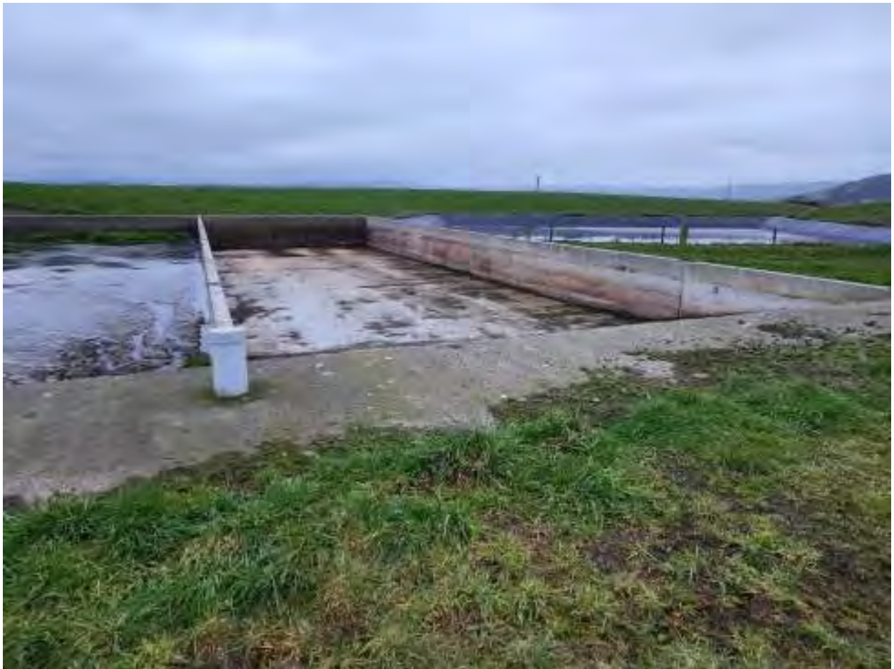
Figure 8 North sludge bed.
