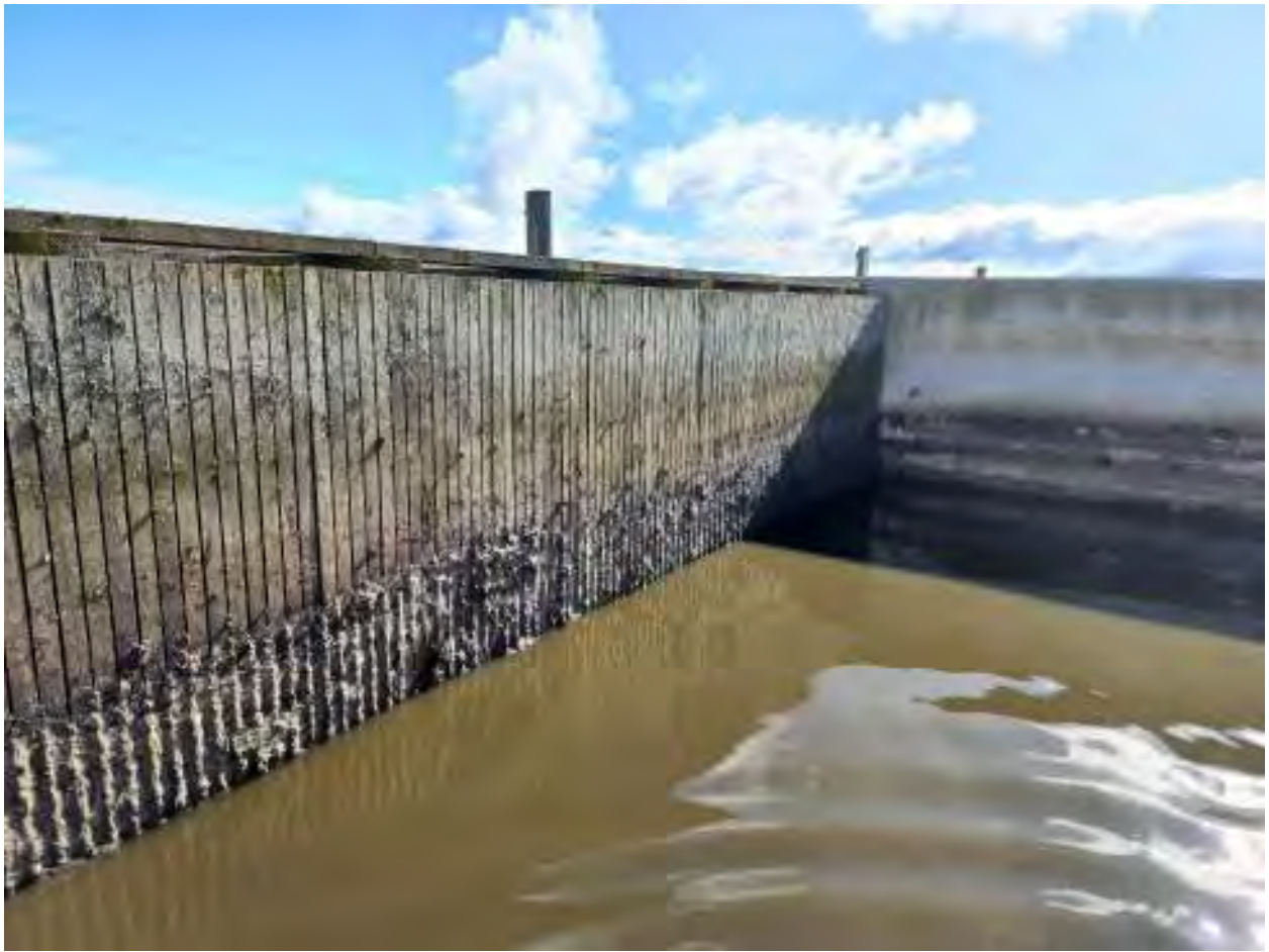
Figure 49 Weeping wall of south sludge bed.
