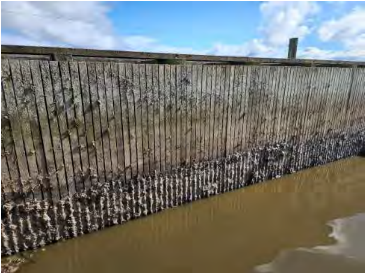
Figure 48 Weeping wall of south sludge bed.
