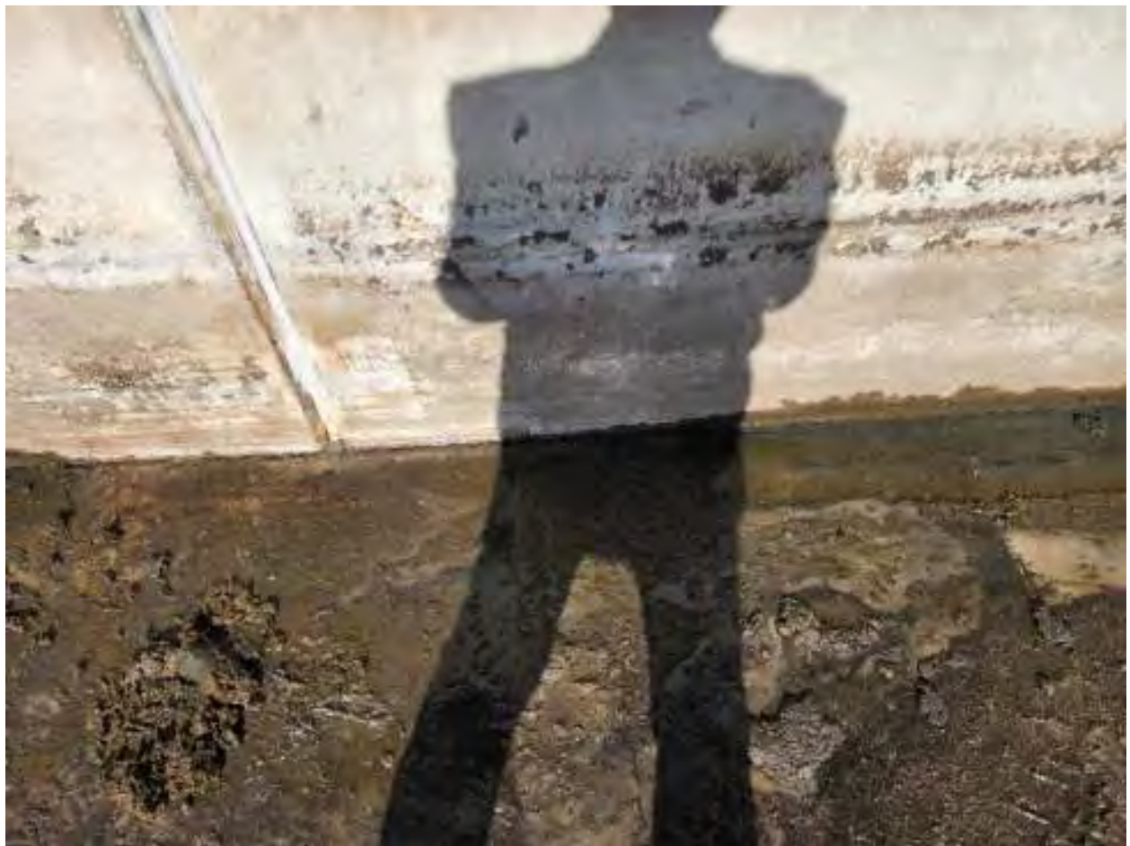
Figure 42 Panel joints of south sludge bed with repaired sealant and edge joint.
