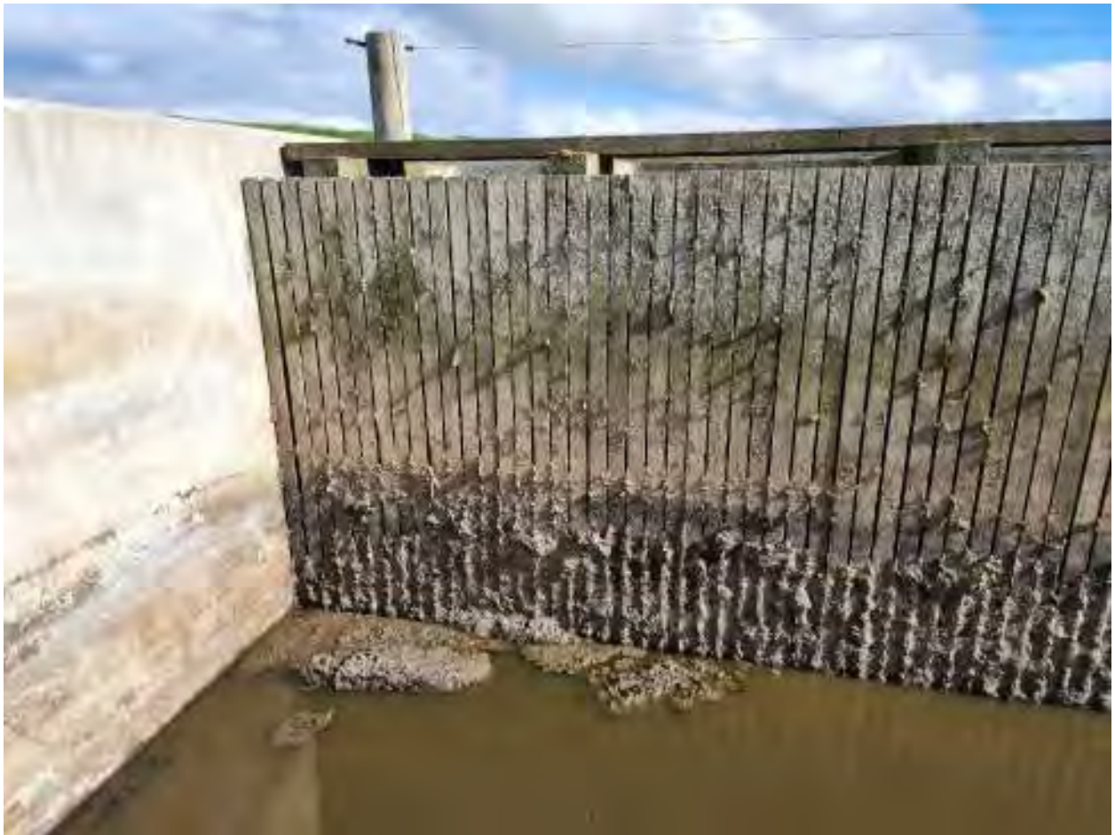
Figure 47 Weeping wall of south sludge bed.
