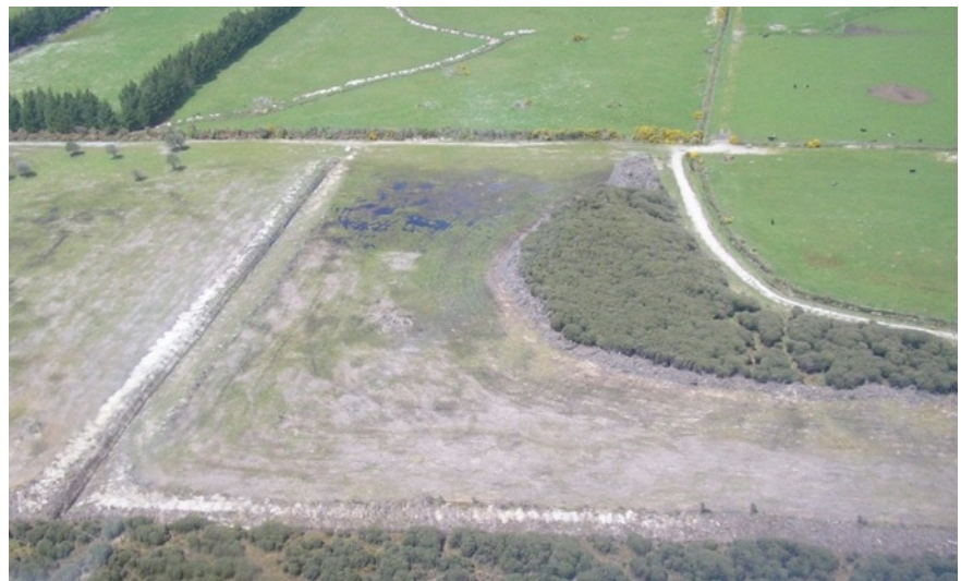
Fig. A1-8. Wetland clearance and drain laying in the lower Waituna catchment, December 2009 (photo: M. Schallenberg).
