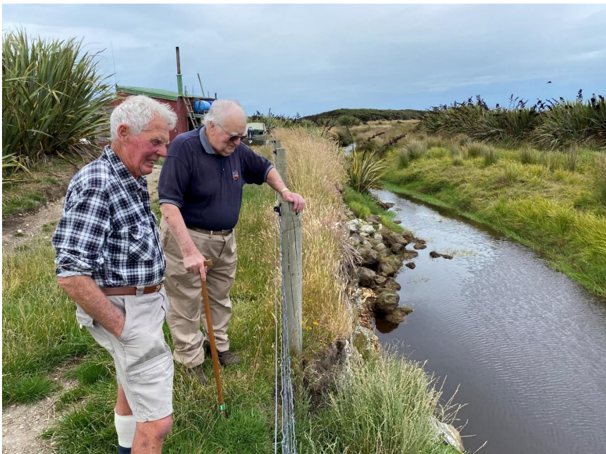
Ray Simms (L) and Lindsay Paddon (R) looking at the Moffat Creek bank erosion in 2022
