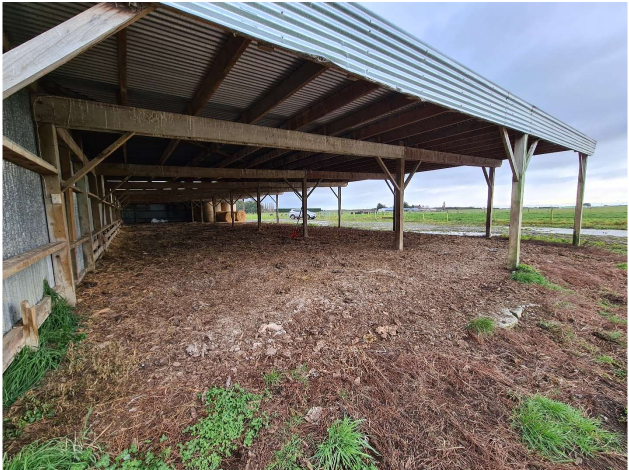
Figure 22 View of the facility looking north-west showing the roof and woodchip spread across the base of the facility.
