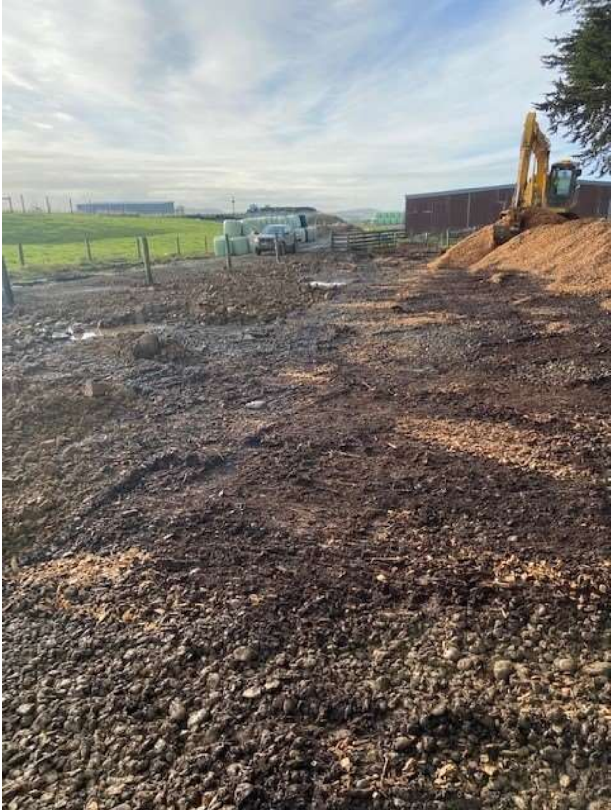
Figure 34 View of north-east corner of the facility looking north-east showing compacted rock base ready for woodchip to be spread (photo supplied by consent holder).
