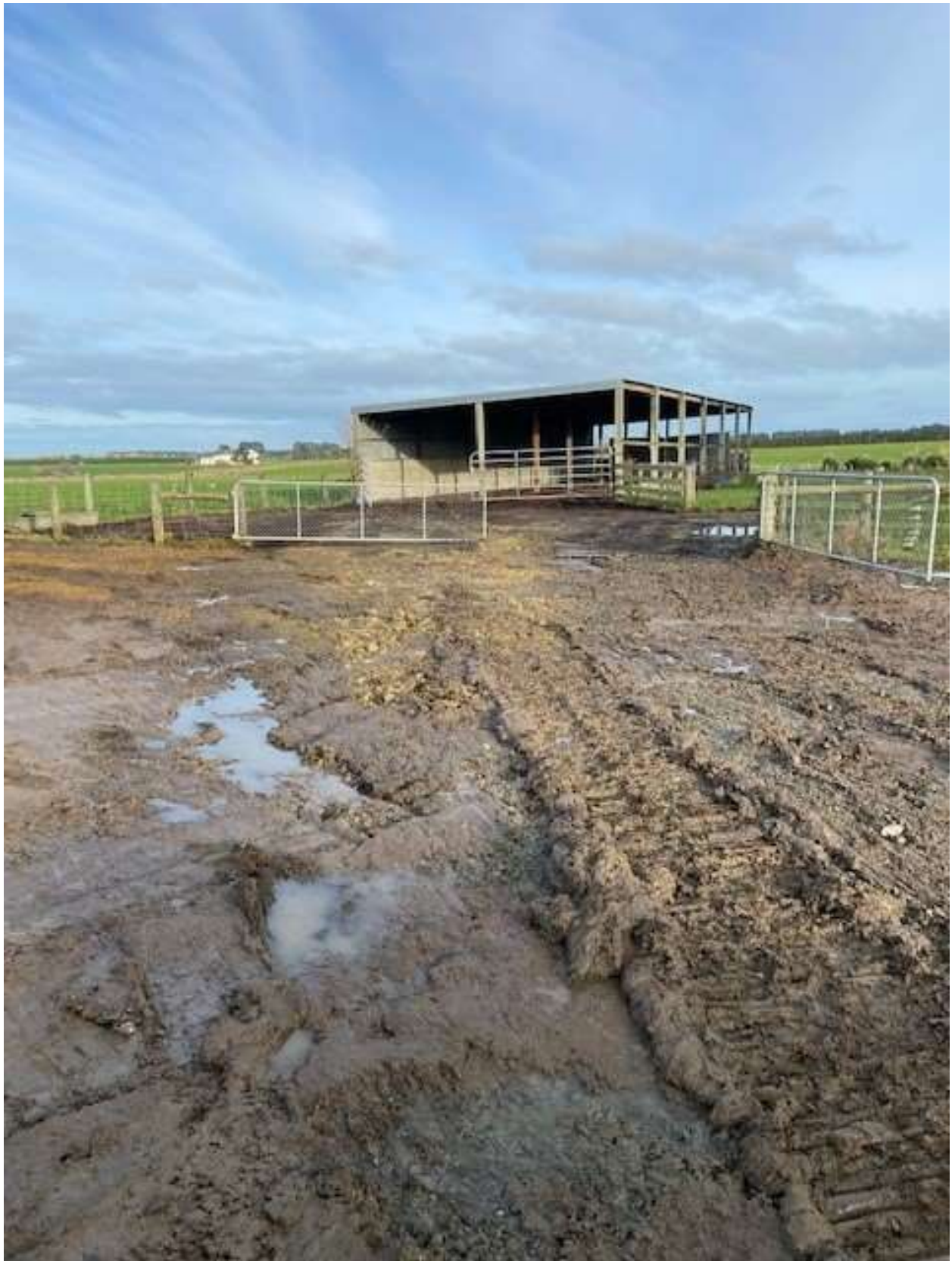
Figure 15 View of the uncovered area looking south-west with the topsoil stripped ready for placement of compacted rock (photo supplied by consent holder).
