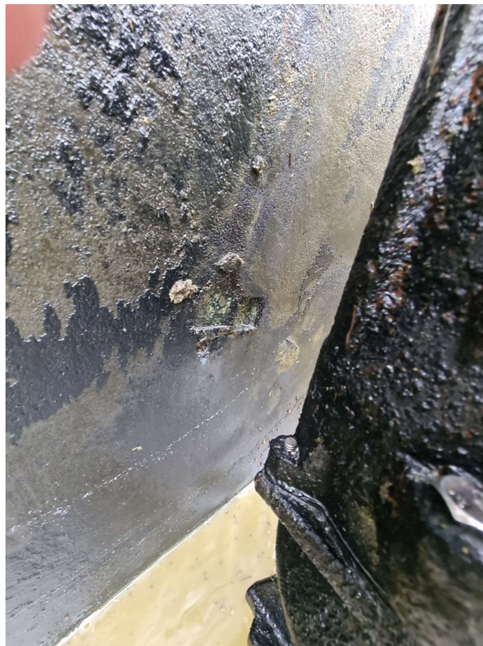
Figure 4 Minor damage behind effluent pump.
