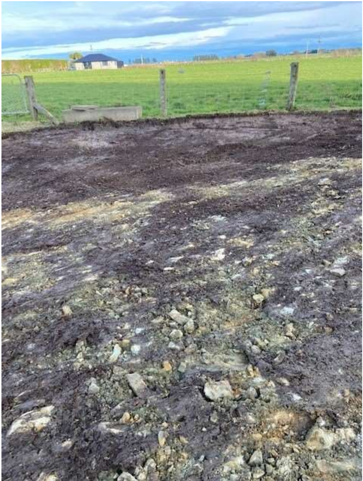
Figure 18 View of the uncovered area looking south with topsoil stripped ready for placement of compacted rock (photo supplied by consent holder).
