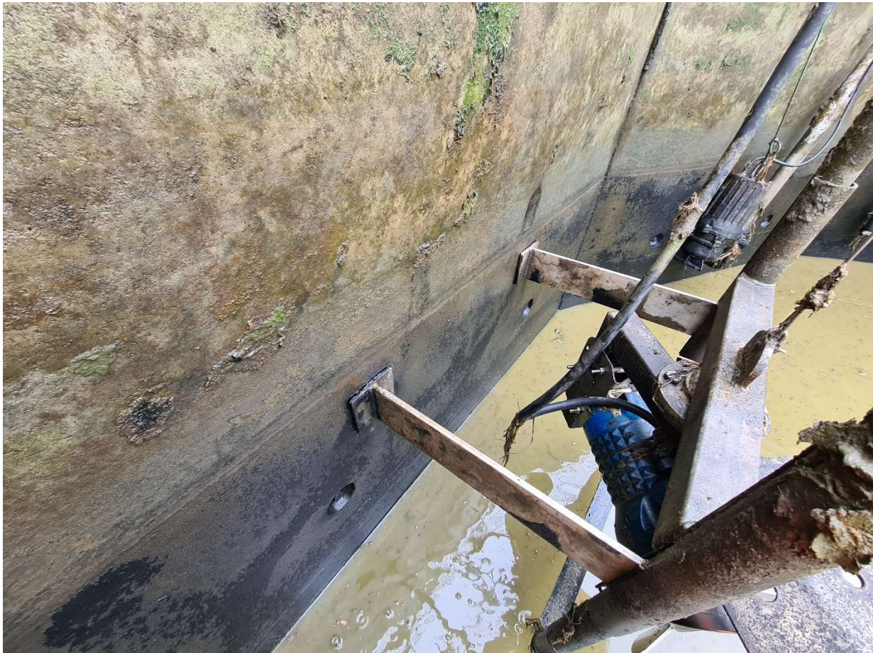
Figure 3 area behind the stirrer- no damage.
