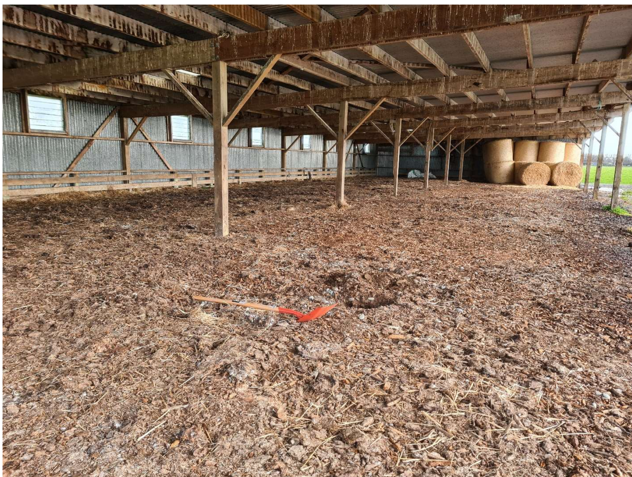
Figure 20 View of the roofed area of the facility looks south-west showing the roof and layer of woodchip across the base of the facility.
