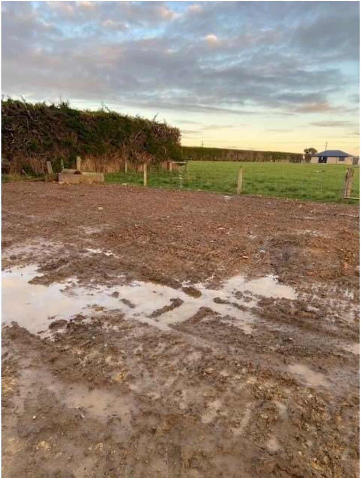
Figure 12 View of the compacted rock base of uncovered area looking south (photo supplied by consent holder).
