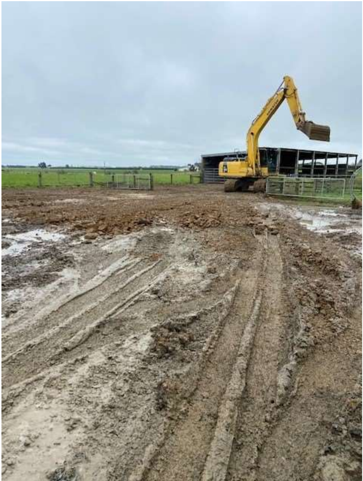
Figure 10 View of the compacted rock base of uncovered area looking south-west (photo supplied by consent holder).
