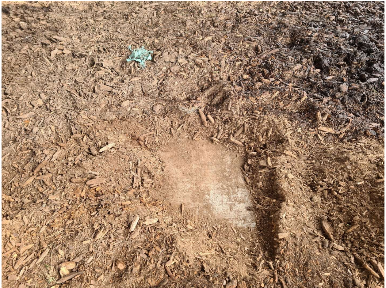
Figure 7 Pit dug in the north half of the roofed area showing layer of woodchip on top of a concrete base.
