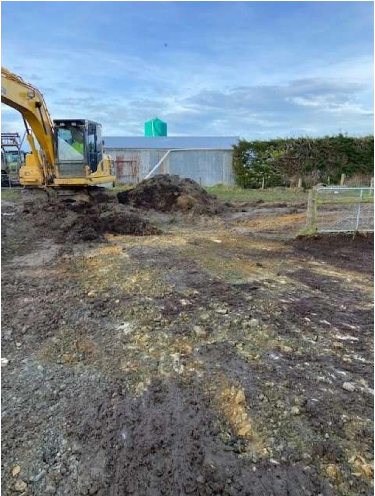
Figure 16 View of the uncovered area looking east with the topsoil stripped ready for placement of compacted rock (photo supplied by consent holder).
