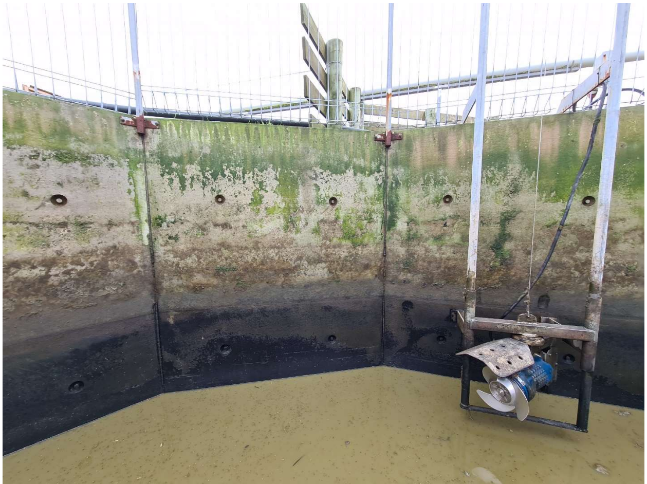
Figure 12 Interior panels of facility and stirrer frame
