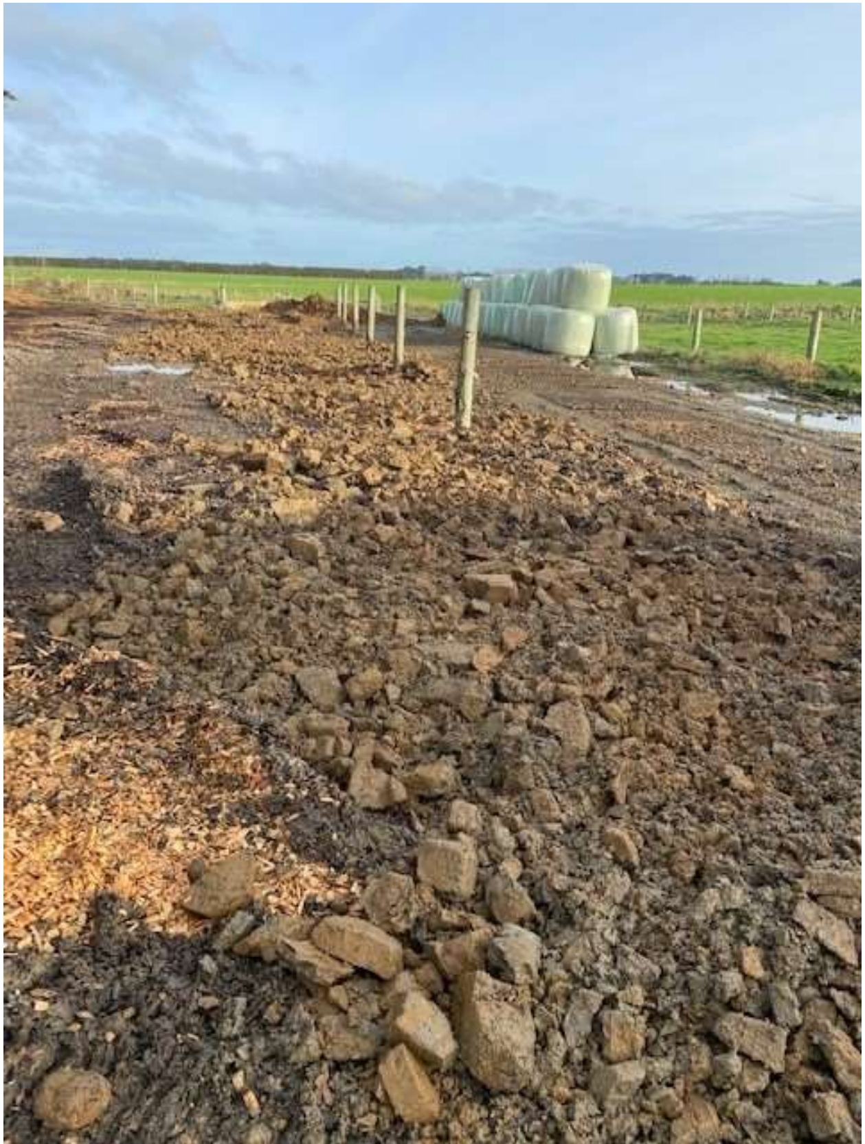
Figure 36 View of north-west corner of the facility looking west showing rock placed on the base of the facility ready to be compacted (photo supplied by consent holder).
