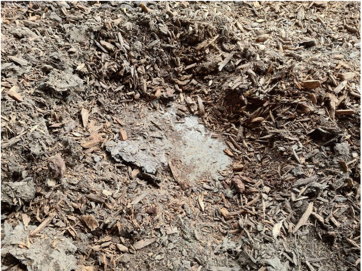
Figure 4 Pit dug in the north half of the roofed area showing layer of woodchip on top of a concrete base.
