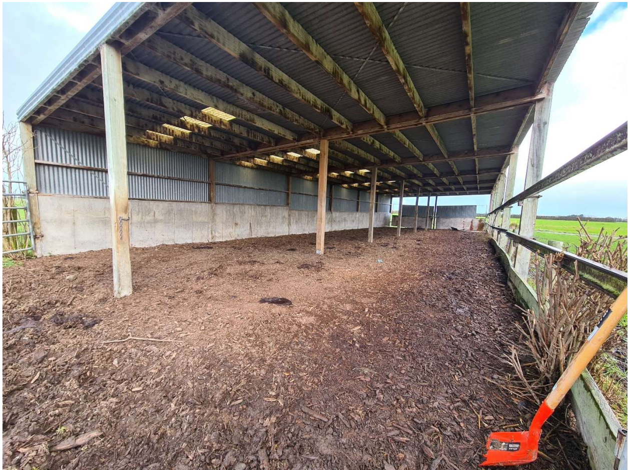
Figure 9 View of the roofed area looking south-west showing the roof and layer of woodchip across the facility.
