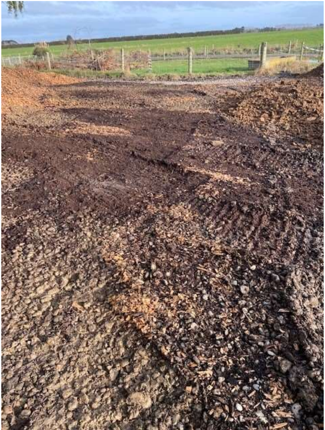
Figure 35 View of facility looking west showing compacted rock base ready for woodchip to be spread (photo supplied by consent holder).
