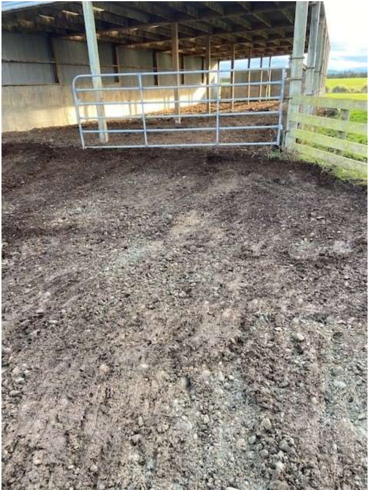
Figure 17 View of the uncovered area looking south-west with the topsoil stripped ready for placement of compacted rock (photo supplied by consent holder).
