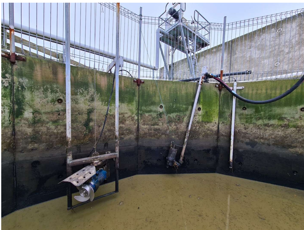
Figure 5 Stirrer frame, effluent pump and float switch
