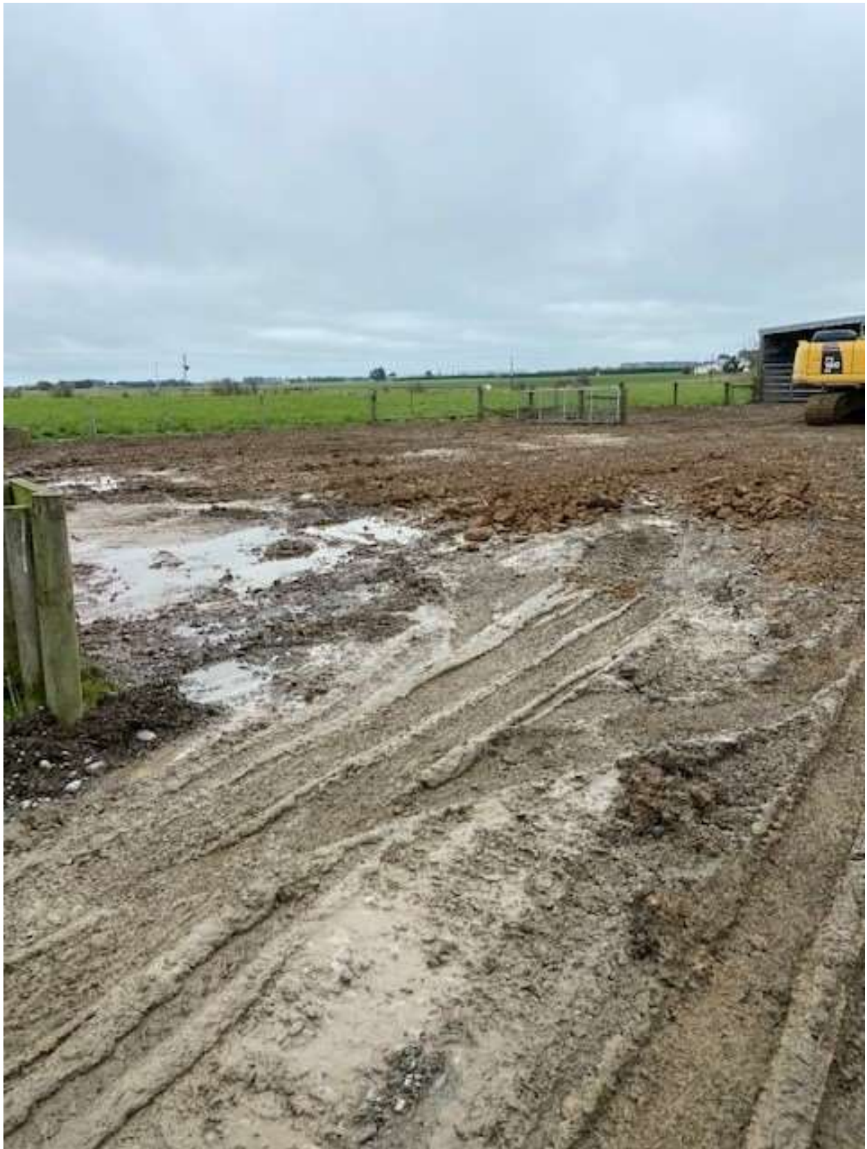
Figure 11 View of the compacted rock base of uncovered area looking south-west (photo supplied by consent holder).
