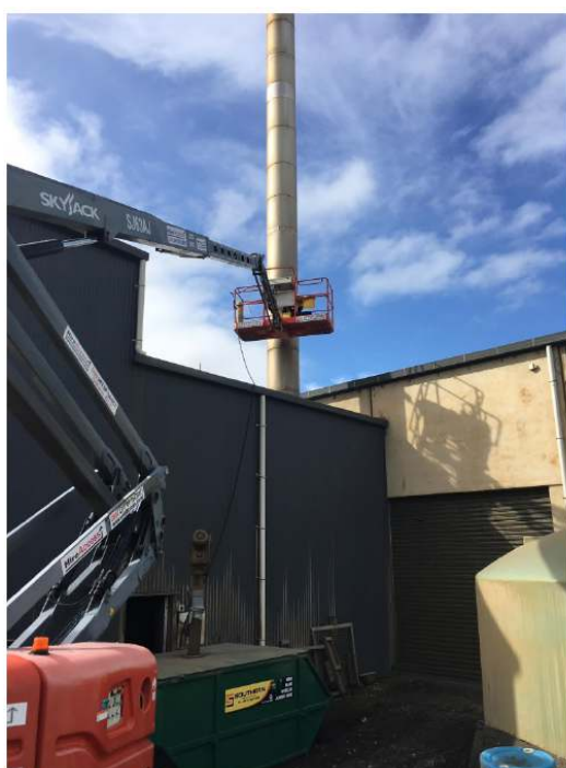
Figure 3-1 4.3 MW Rendering boiler stack sampling location.
