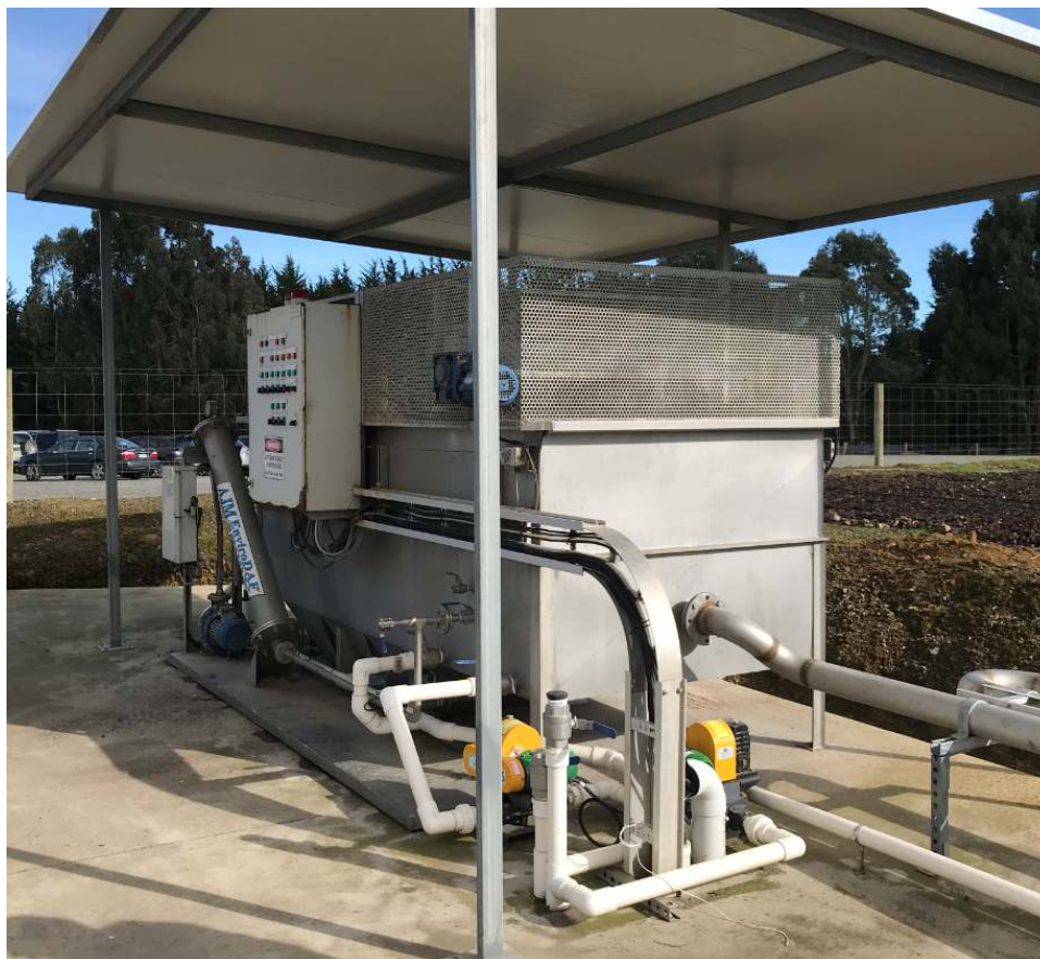
Figure 2-5 Rendering plant liquid waste (Stickwater) DAF plant
