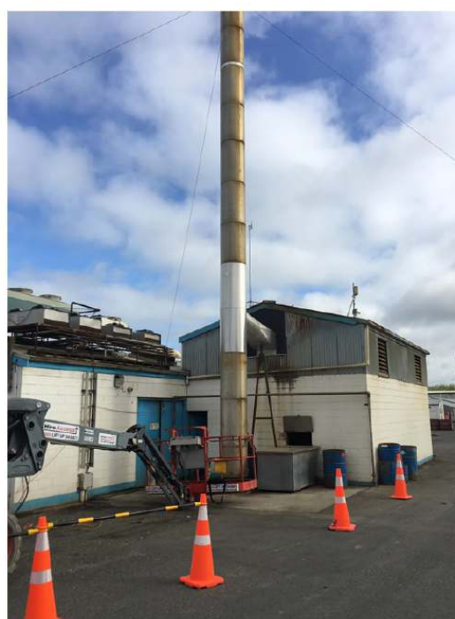
Figure 3-2 2 MW Hot Water boiler stack sampling
