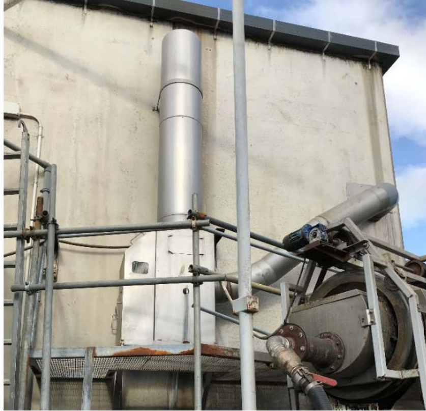
Figure 2-3 Hydrolyser scrubber and vent
