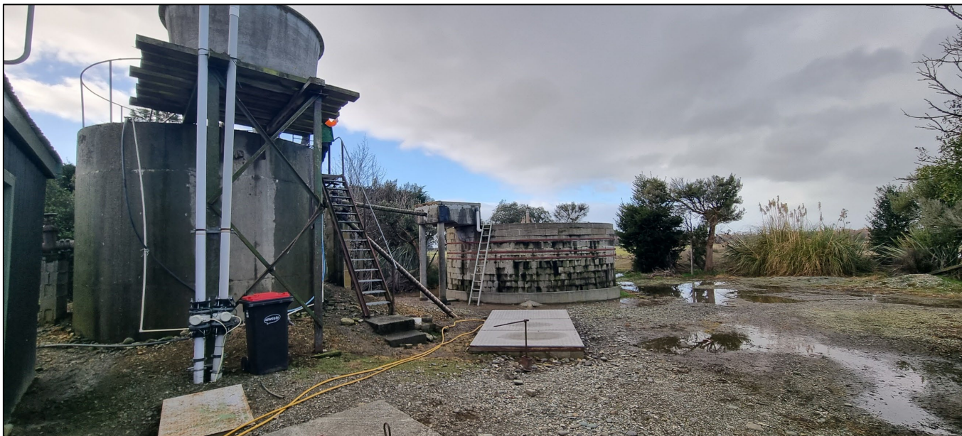
Figure 24 Imhoff tank (left tank)
