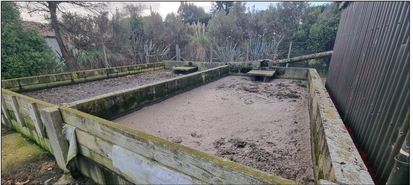
Figure 26 Sludge drying beds
