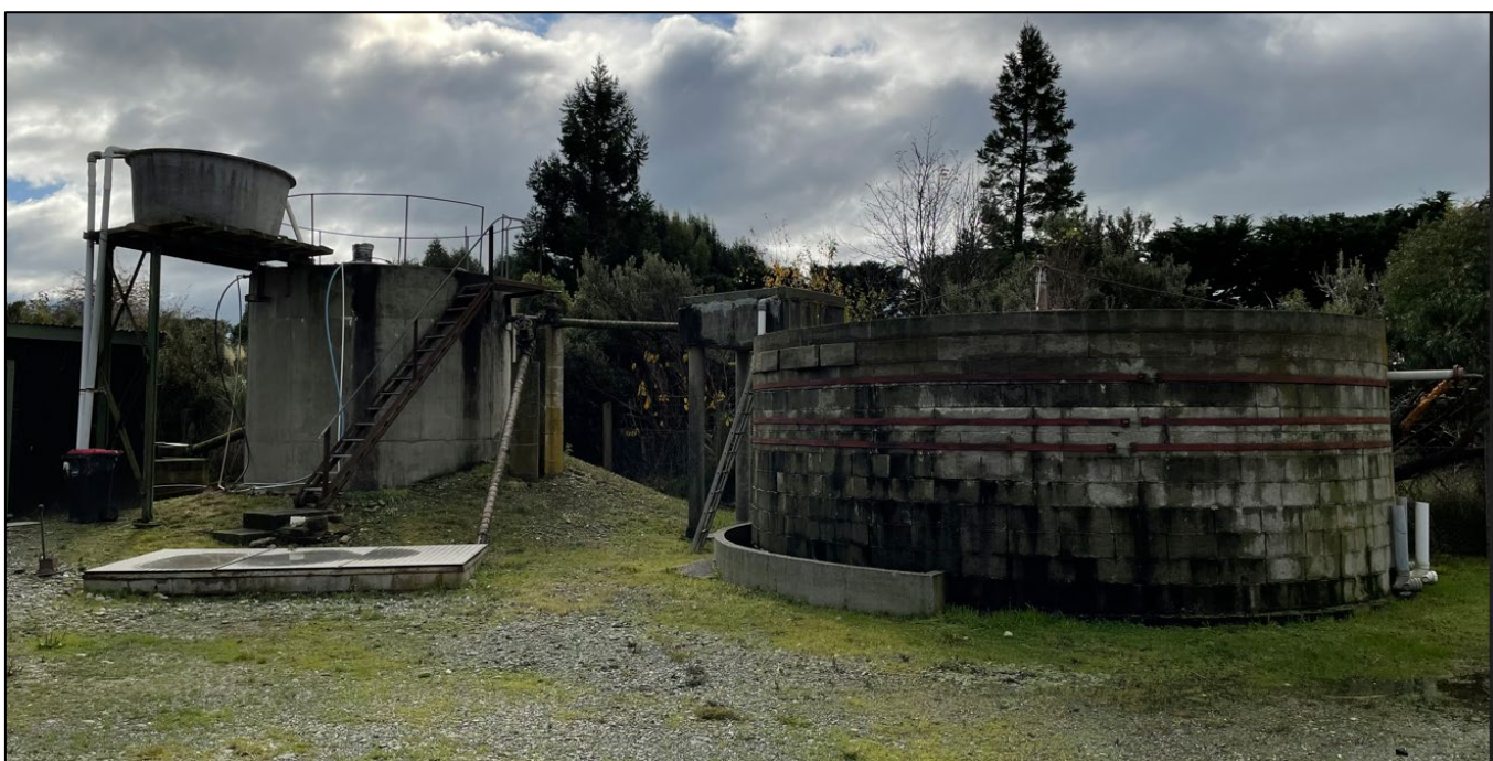
Figure 25 Weir tank situated on ground level attached to trickling filter
