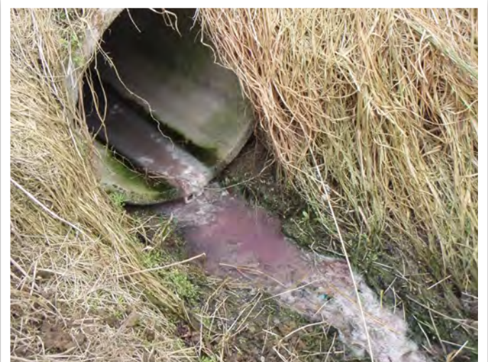
Effluent from a failed septic tank seeps through a culvert.
