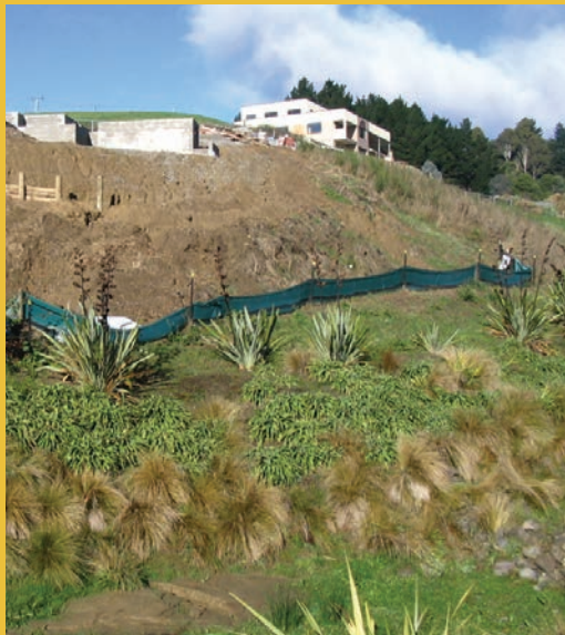
Silt fence and vegetation buffer
