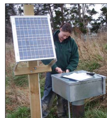
An ES Environmental Technical Officer inspects one of the Waimea Plains Aquifer groundwater level sites.
