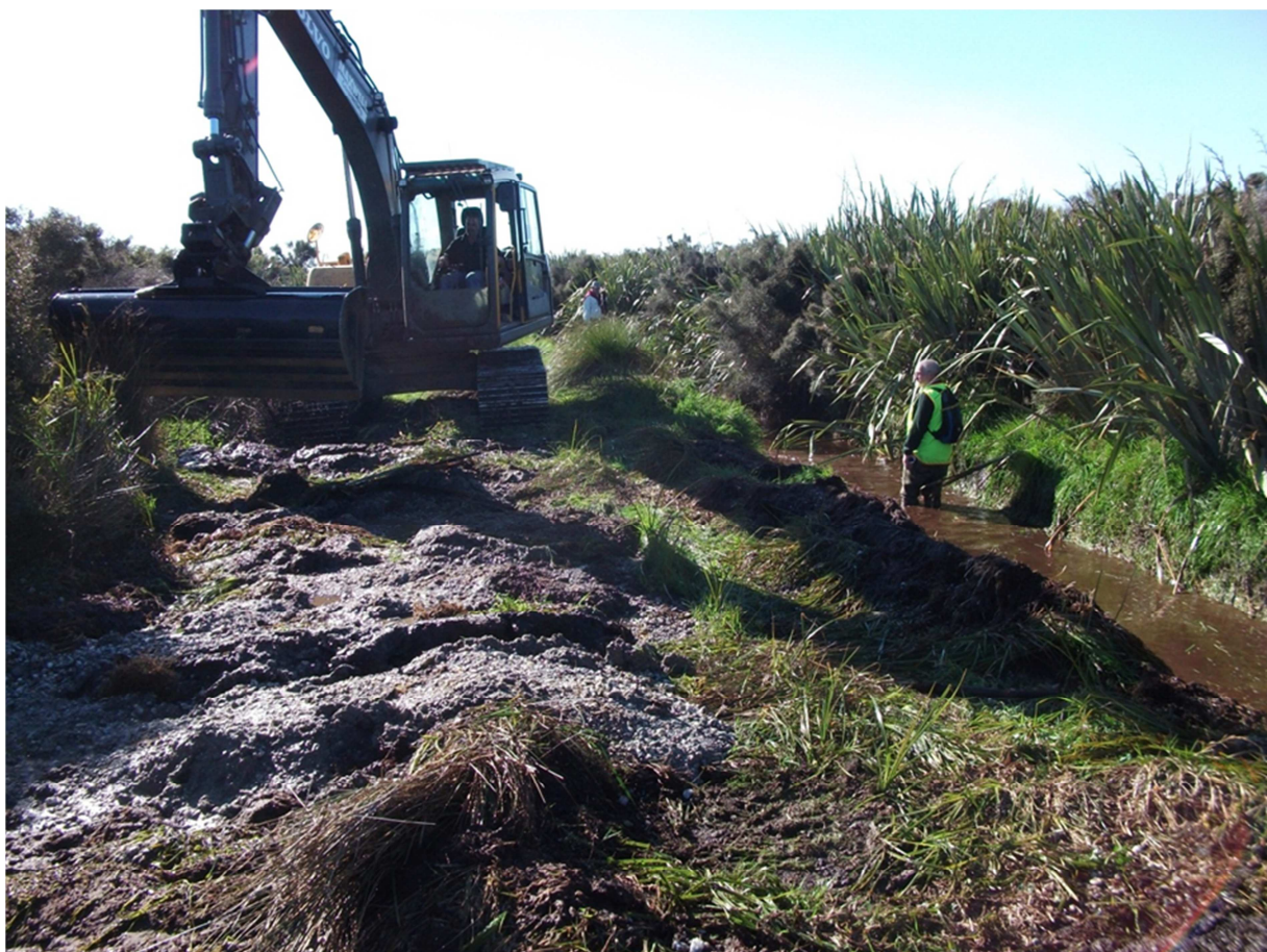
Figure 3-1: Digger clearing sediment from Carrans Creek in the Waituna Lagoon catchment. Photo: Katrina Robertson (Environment Southland).
